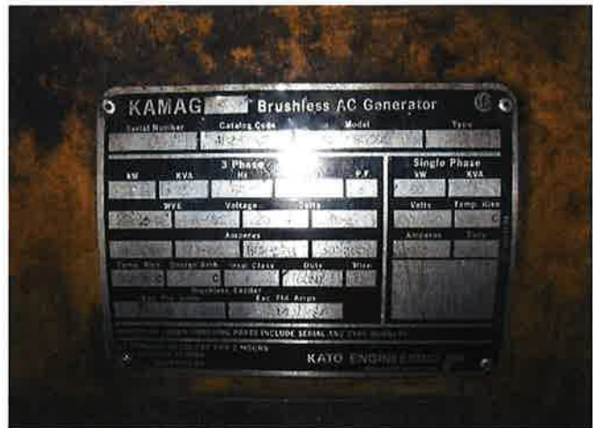
100 kW AC generator
