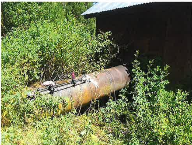
22 inch diameter steel penstock
