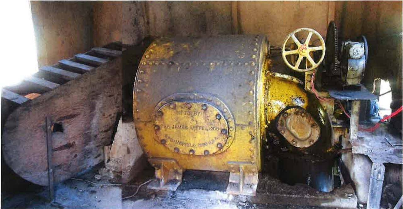
Panoramic view inside the building that houses the turbine and generator
