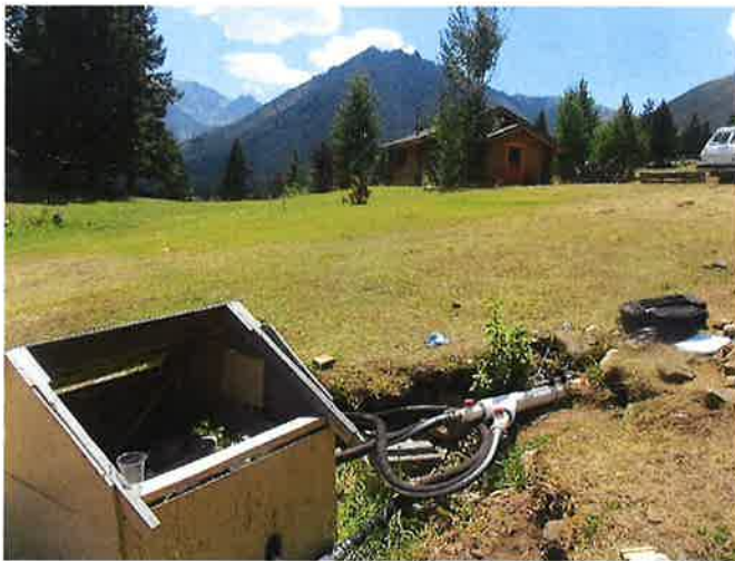
4 inch piping and valves/ lines for two turbines
