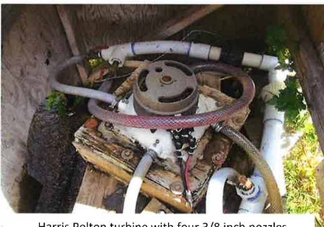
Harris Pelton turbine with four 3/8 inch nozzles
