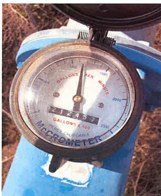
Well 2 Flow Meter
