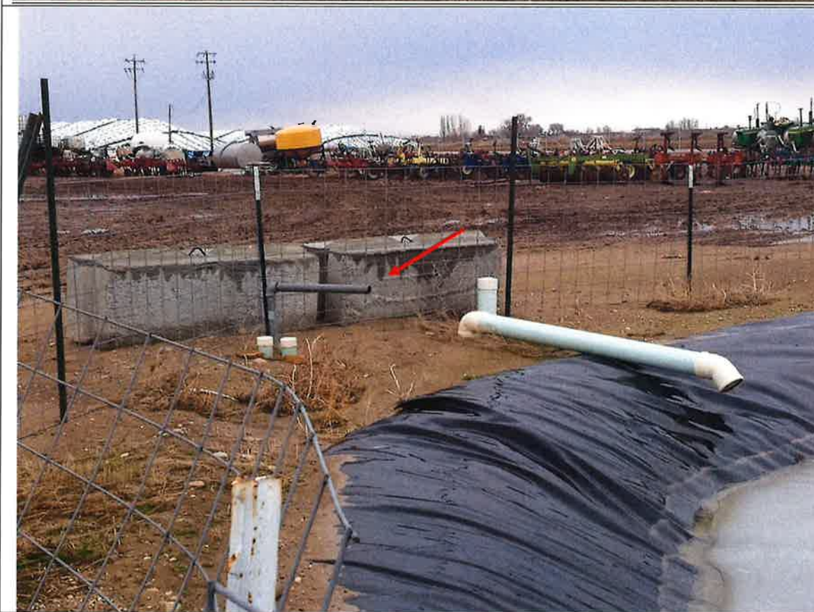
2" galvanized pipe fills the pond as necessary from the well.
