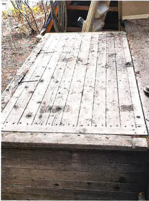
Figure 3 The housing for the pump, which could be locked by the watermaster if necessary.
