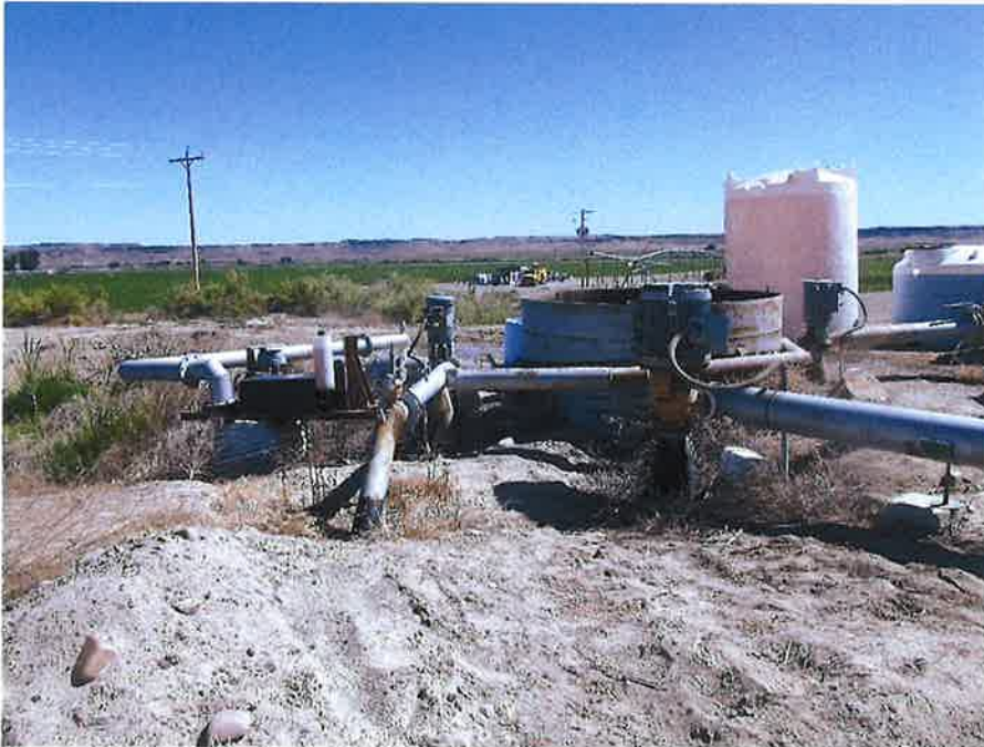
Photo 2: Diversion and Relift Pumps
