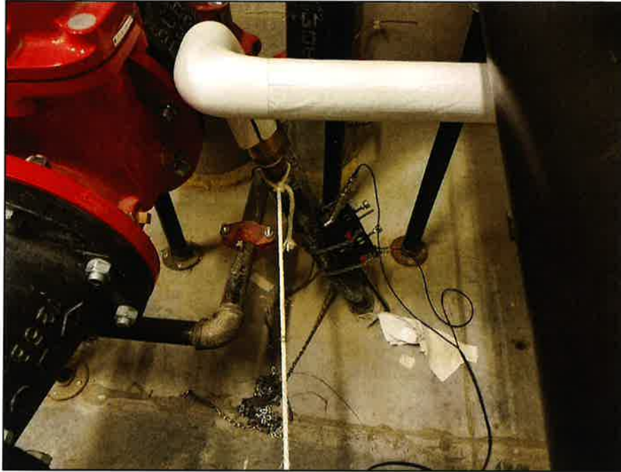
Figure 3: Flowmeter transducers mounted on 2-inch plastic pipe entering facility from well.
