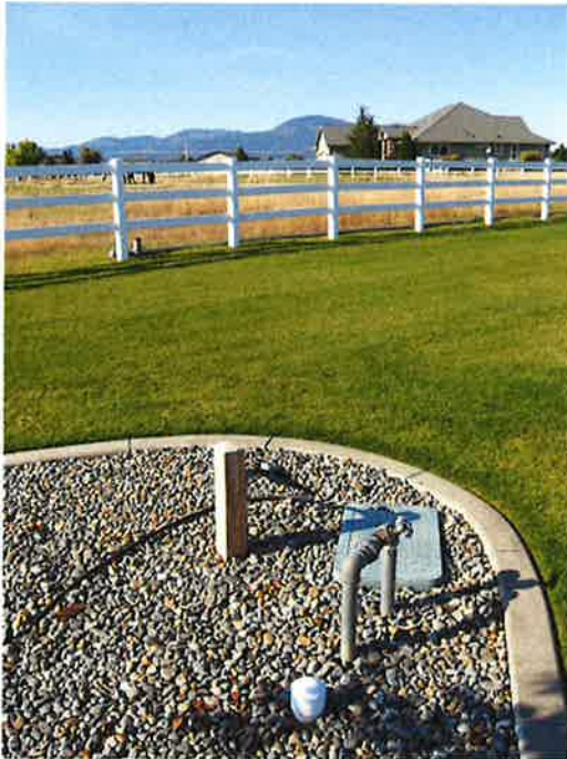
BIG SKY ESTATES IRRIGATION PIPE ON ONE PARCEL
