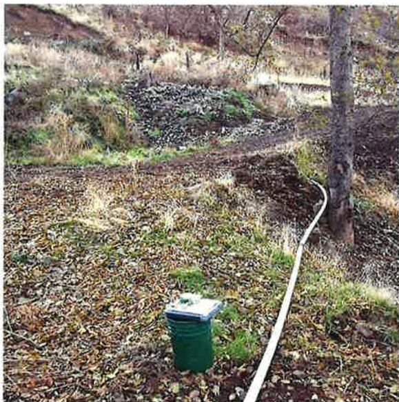
Spring 4 (rocky area) with water line under road. Gravity Feed to portion of Irrigation POU near house and to pond.
