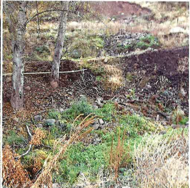
Spring 4 Water Line. View south across road to hill side.
