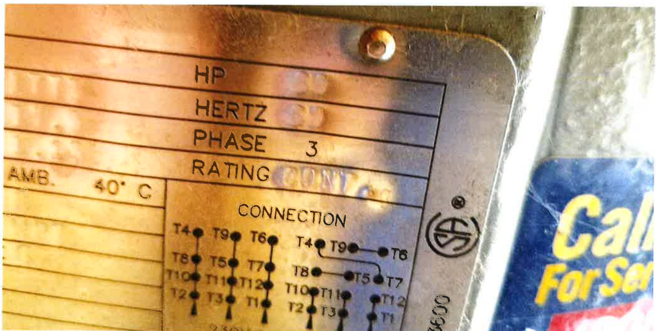
Close-up of nameplate on south 60-hp motor.
