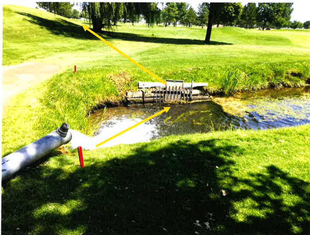
Temporary mainline discharging to golf course pond system. Headgate and trash rack to downstream ponds in background. Irrigation District water enters from right side. Mixed water flows in buried pipe approximately 200 feet to reach intermediate pond to the north.
