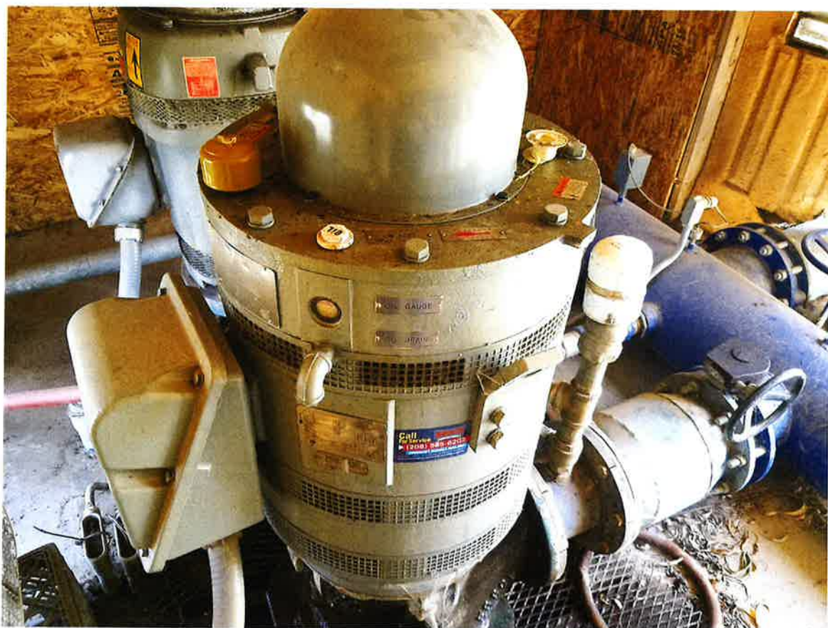
Vertical turbine pressure irrigation pumps. Both motors are 60 hp.
