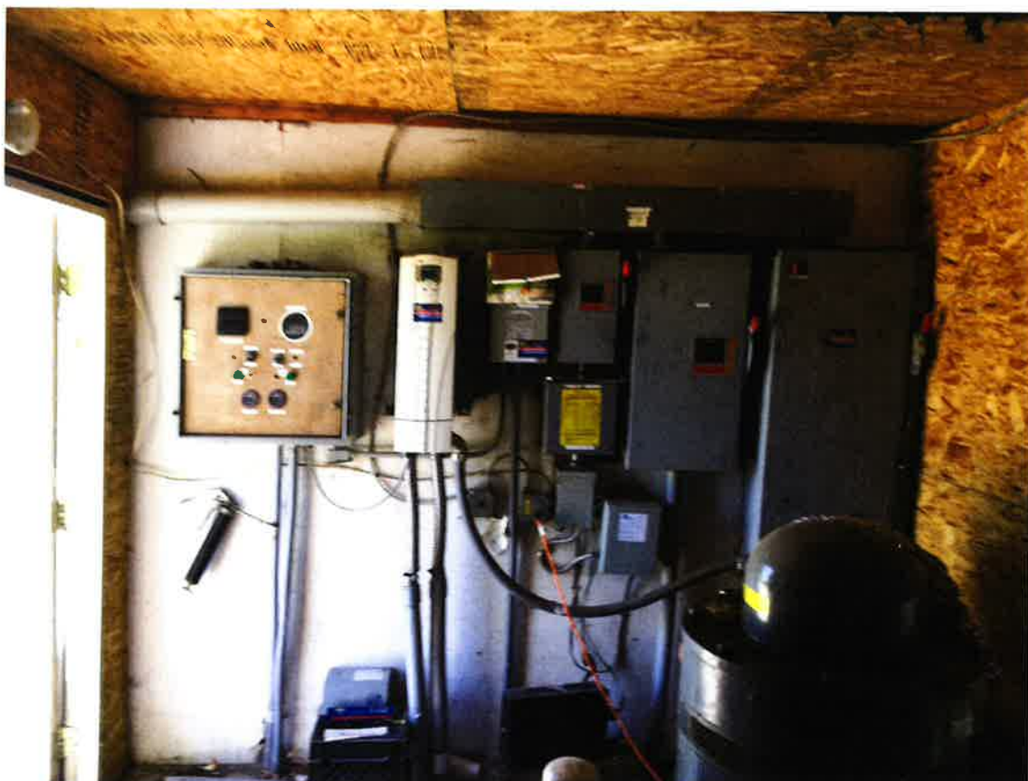
Pressure irrigation pump station motor controls
