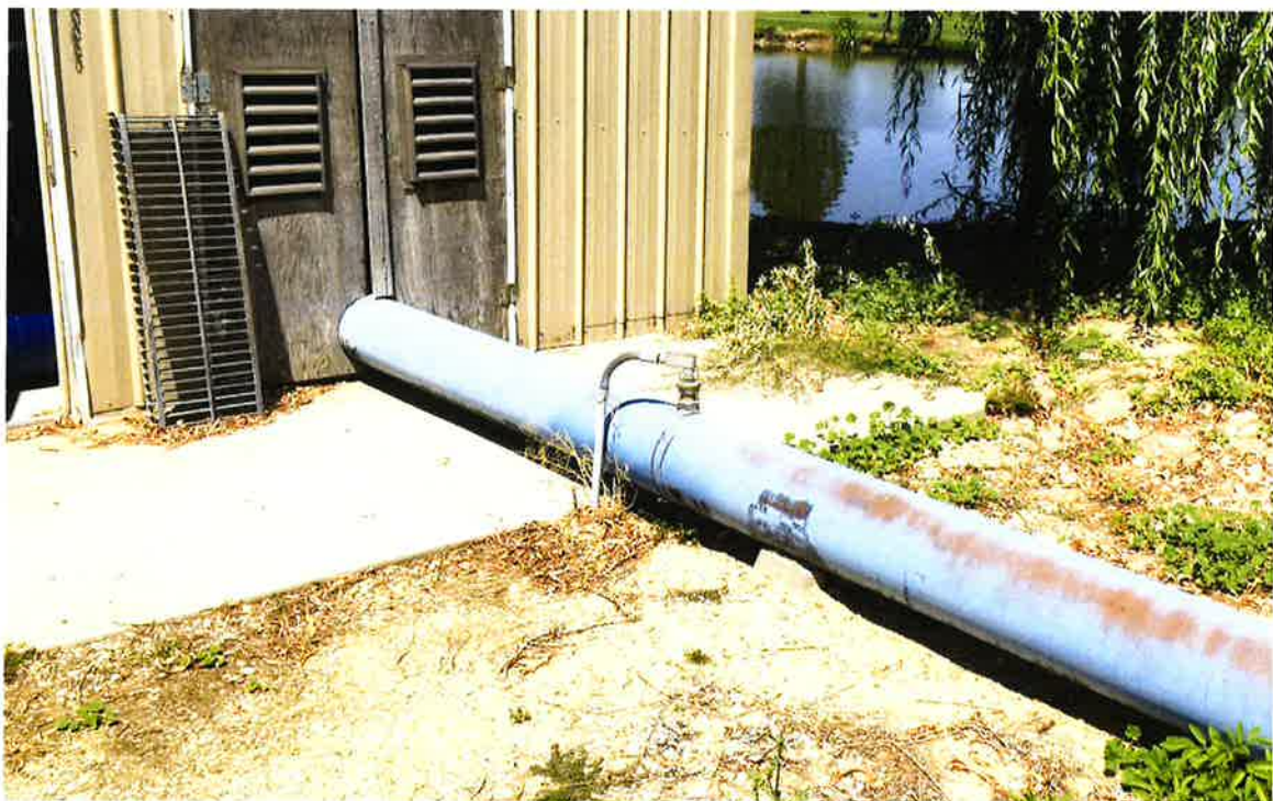
Discharge piping from pressure pump station. Insertion flow meter for Maxicom irrigation controls is visible.
