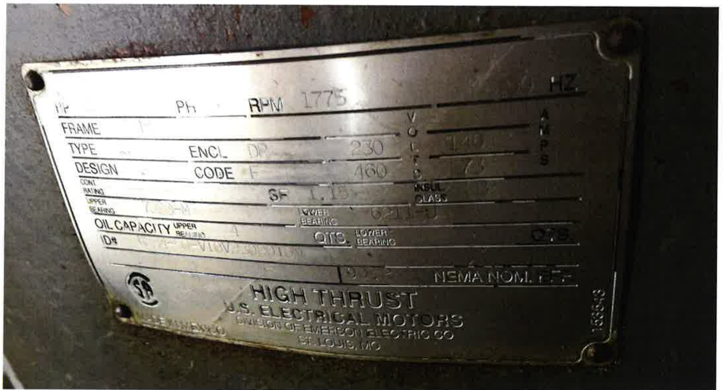
Nameplate on north 60-hp motor.
