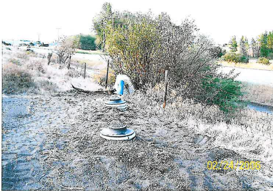
Terminus of the Sam's Hollow mitigation pipeline.
