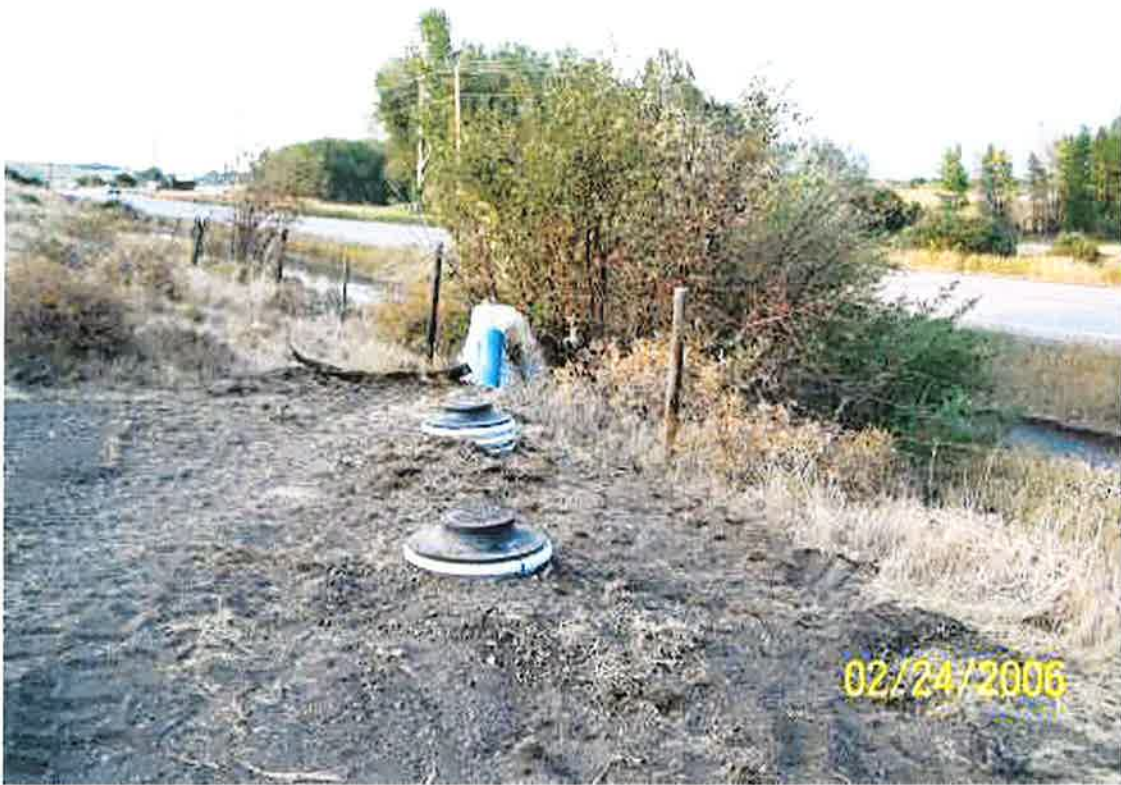
Terminus of the Sam's Hollow mitigation pipeline.
