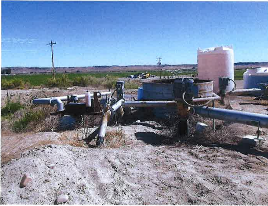
Photo 1: Pump diversion from wastewater
