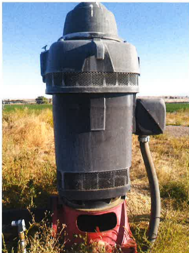
Figure 1. The 150 hp max vfd motor running the pump, which is set at 262 ft BGS.
