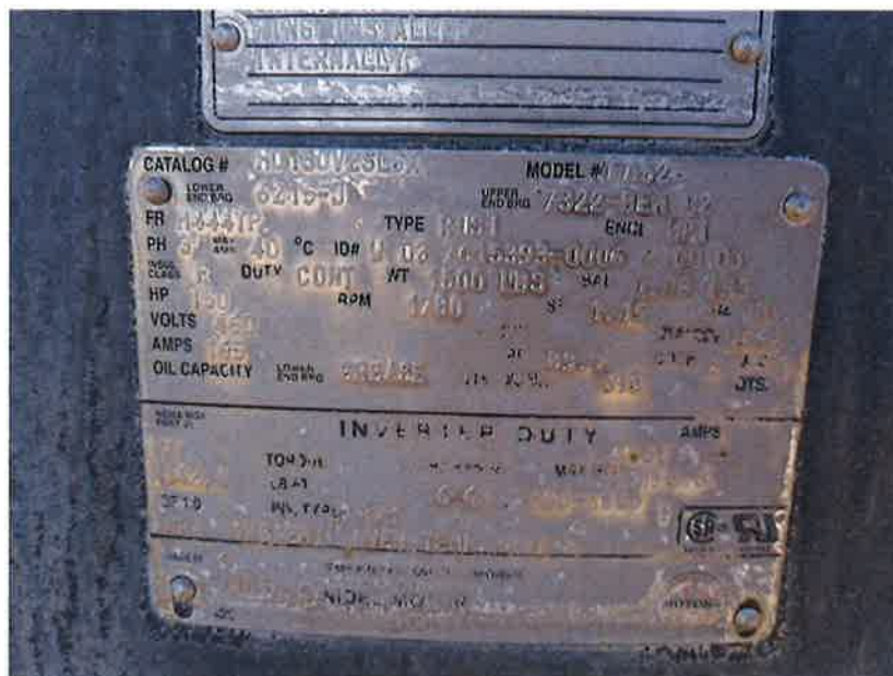
Figure 2. The specification tag for the electric motor.
