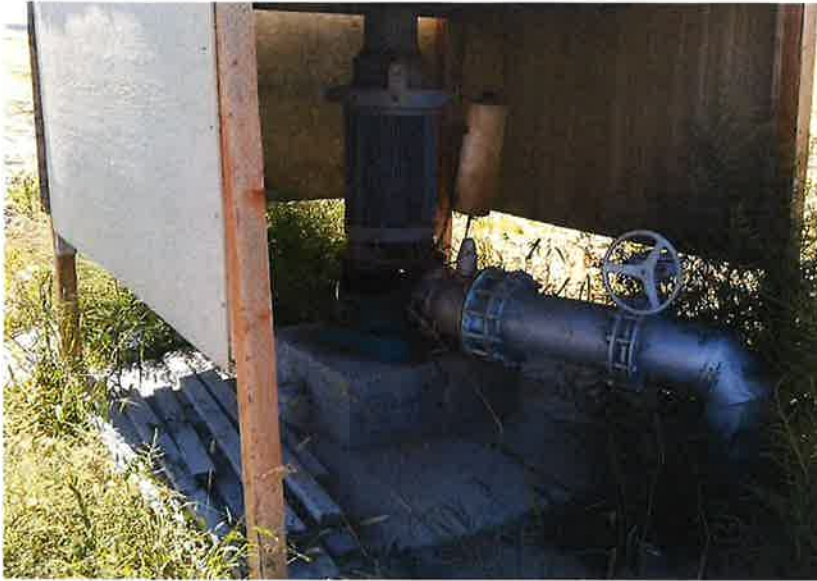
Figure 1. The well with a 100-hp motor. Water is moved through a 10-inch line from the well to the open discharge.
