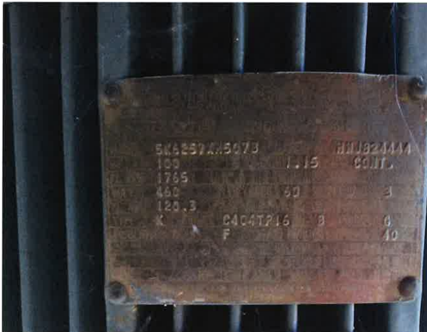
Figure 2. Tag showing the specifications for the GE motor.
