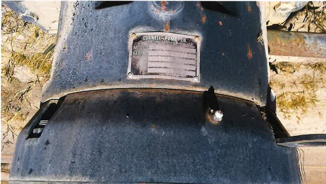
Figure 6. The spec tag for the booster pump used to charge the pivot.
