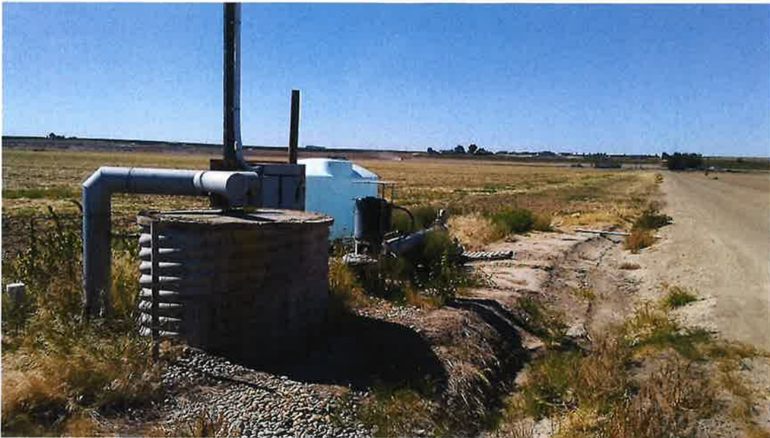
Figure 5. Open discharge from 10-inch line to vault.
