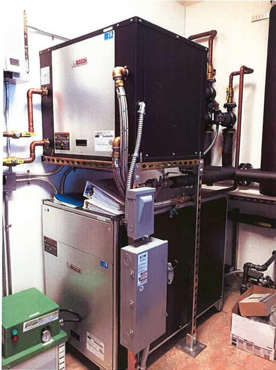
Figure 8: Bosch 6 ton heating unit (top) and 10 ton heating and cooling unit (bottom) associated with heating and cooling uses for residence.
