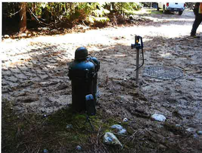
HUCK BAY Well 2 Vault cover
