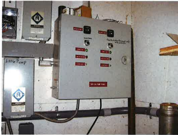
HUCK BAY Pump house Controls
