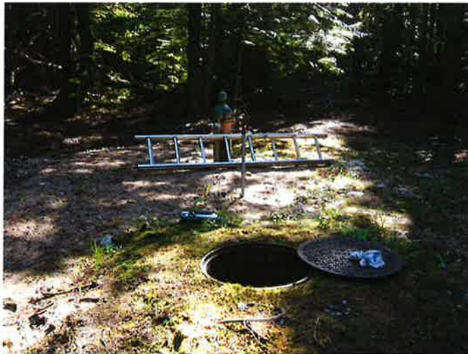
HUCK BAY Well 1 Vault
