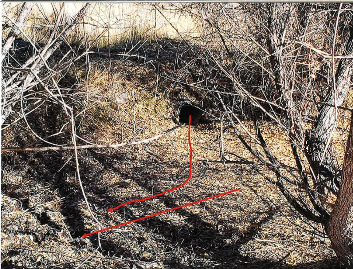
Corrugated pipe delivers surface water to the pond system. The ditch connects all the ponds together. Conveyance from Pond A to B
