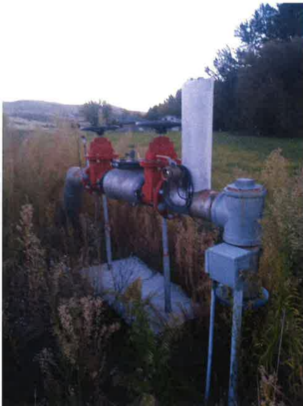
Figure 2. 10" steel mainline from the well to risers and to the gated pipe.
