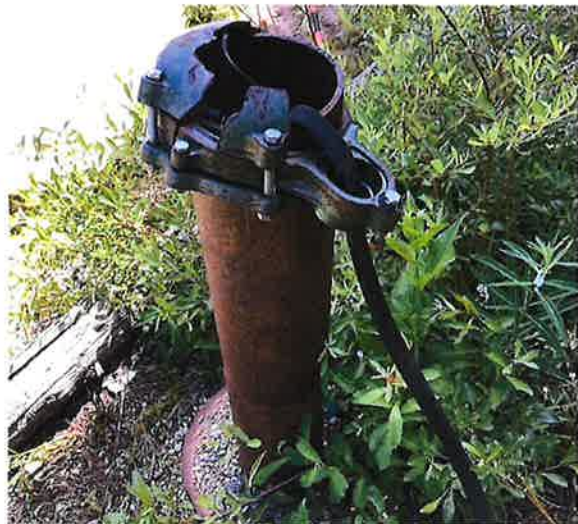
Photo 24. Mid Mountain Well 2 (6 inch diameter). Note the broken cast iron well cap. Tamarack representatives ordered a replacement cap for this well while we were on site. No Tag on well, but well records indicates that the Tag Number is D0047295, which was welded on the Mid Mountain Well 1, for which no tag was issued.
