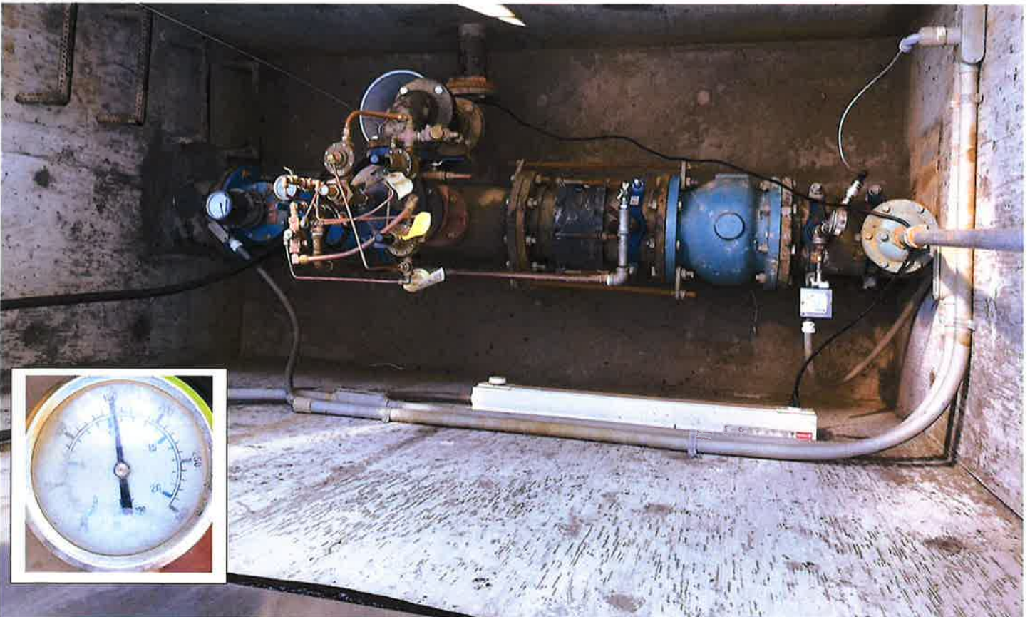
Photo 13. View inside the well 5 vault with various piping, valves, and gages. Pressure gage reading during operation at capacity was 150 PSI. The horsepower associated with this pump is unknown.
