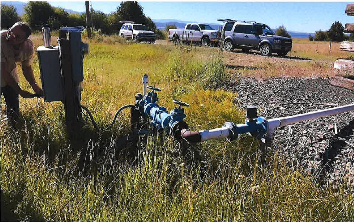
Photo 2. Well 1 valves, flow meter, and piping to storage tank. Note the broken pipe in front of flow meter. Not operable.
