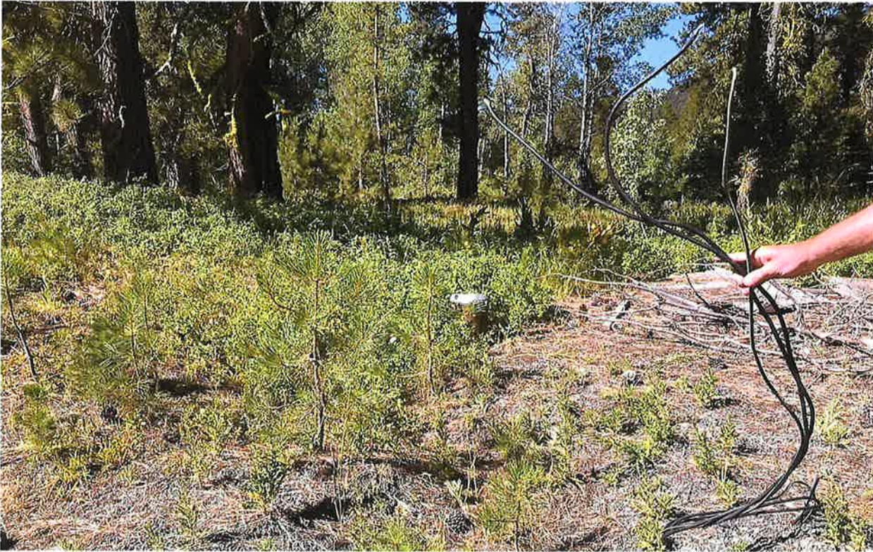
Photo 5. Well 9 was not operational. The power supply was completely disconnected as shown in the photo.
