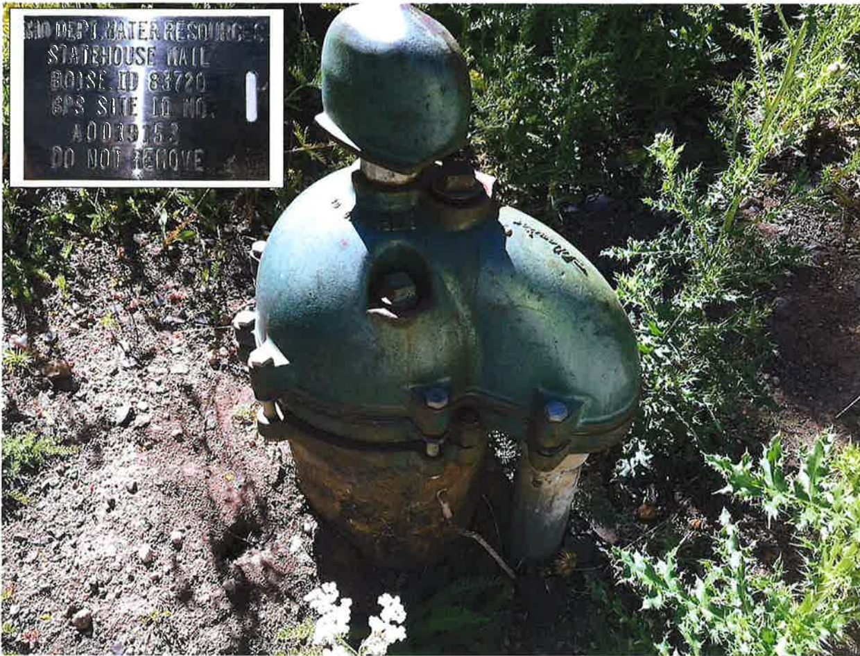
Photo 7. Well 4. This well is for potable water only. The well did not have a tag number, but the well log indicates that well tag D0029486 was issued for this well. We added well tag A0019153 to the well.
