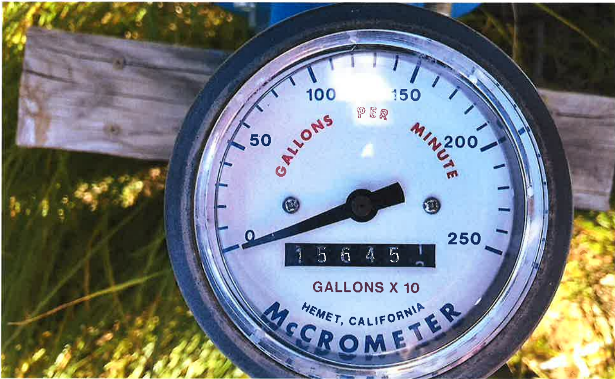
Photo 3. Mechanical McCrometer flowmeter with volume totalizer (1,564,520 gallons = 4.8 acre feet) and instantaneous flow rate. Due to age and climate conditions this flow meter is likely not accurate or functional.
