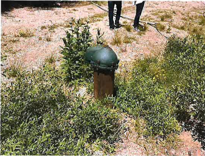
Photo 23. Mid Mountain Well 1 (8 inch diameter). Not connected. The tag number welded on this well is D0047295, which was issued for Mountain well 2. The well drilling application shows that this well was drilled as a drill and fill and no tag was issued.
