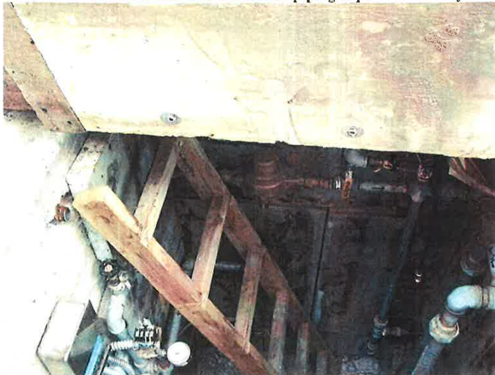
Photo 1. Well #1 flowmeter and connection piping to potable water system.
