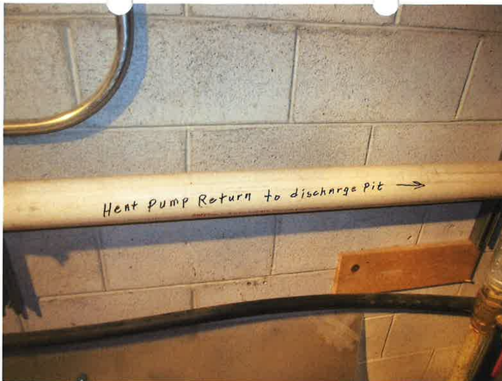
Return line from heat pump system to subsurface discharge pit
