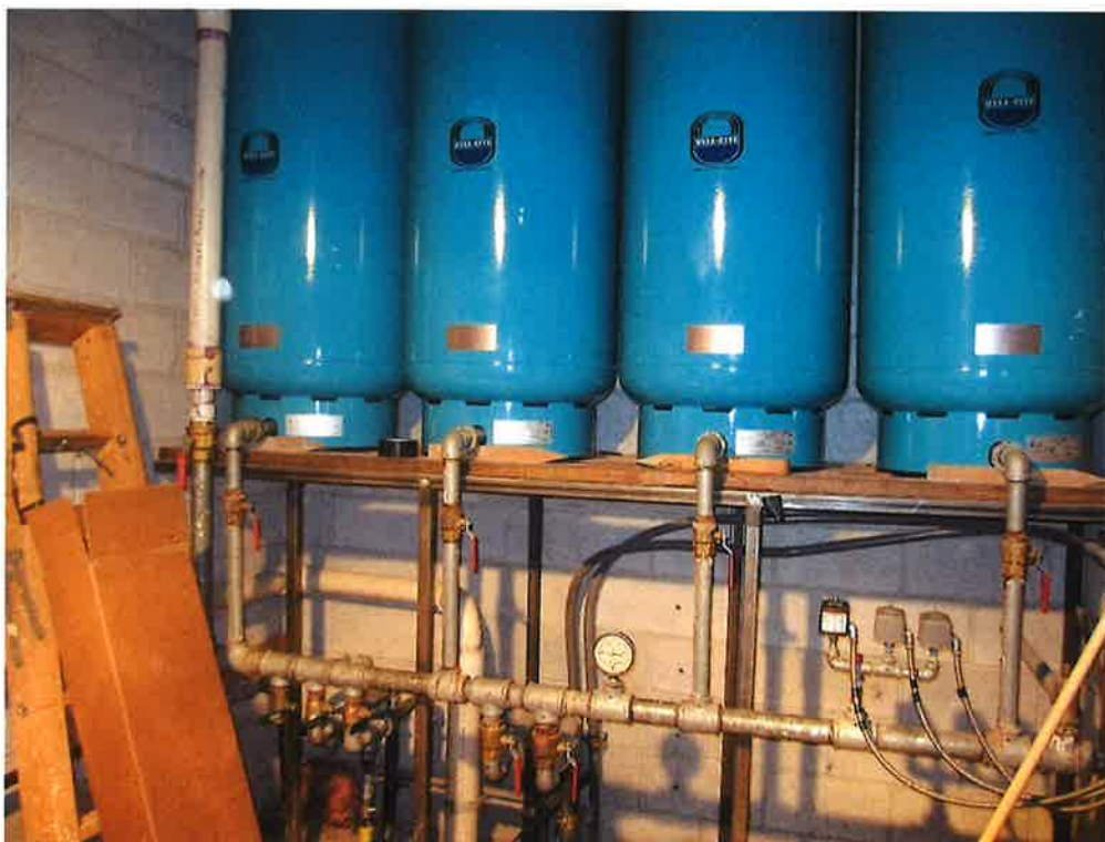
Plumbing for heating/cooling system inside building
