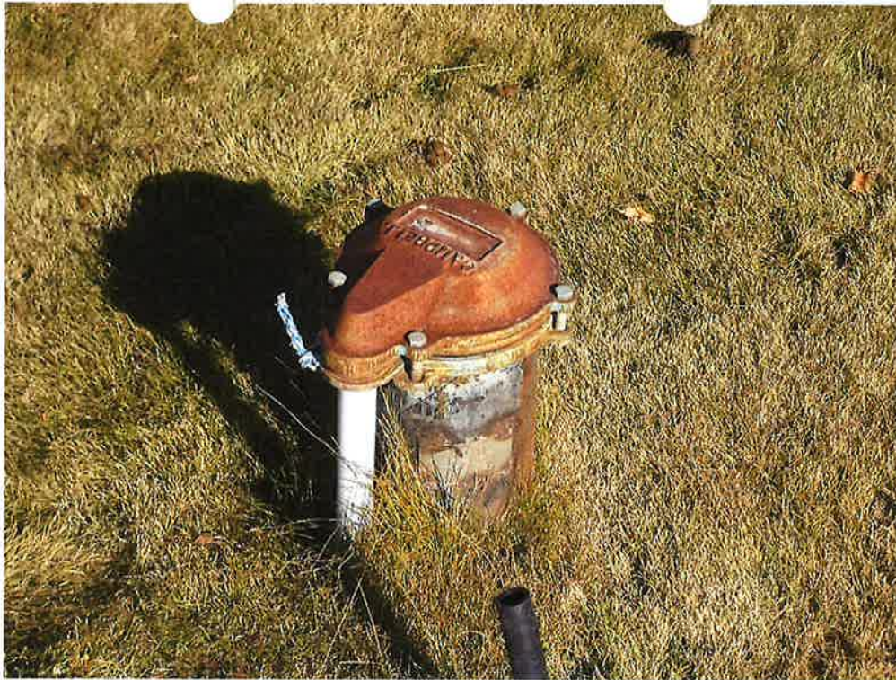
Well nearest building – Tag #D0008368
