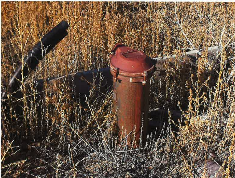
Well in southeast corner of parking lot - Tag #D0008369
