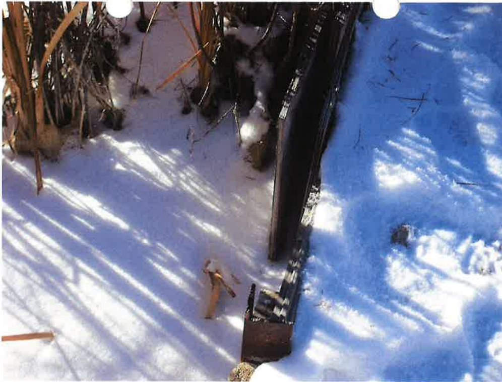
Headgate at the point of diversion
