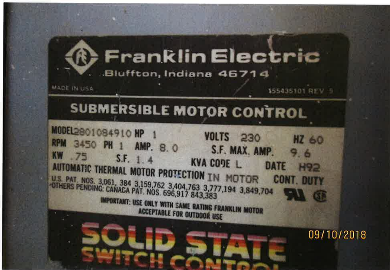
1hp pump in well.
