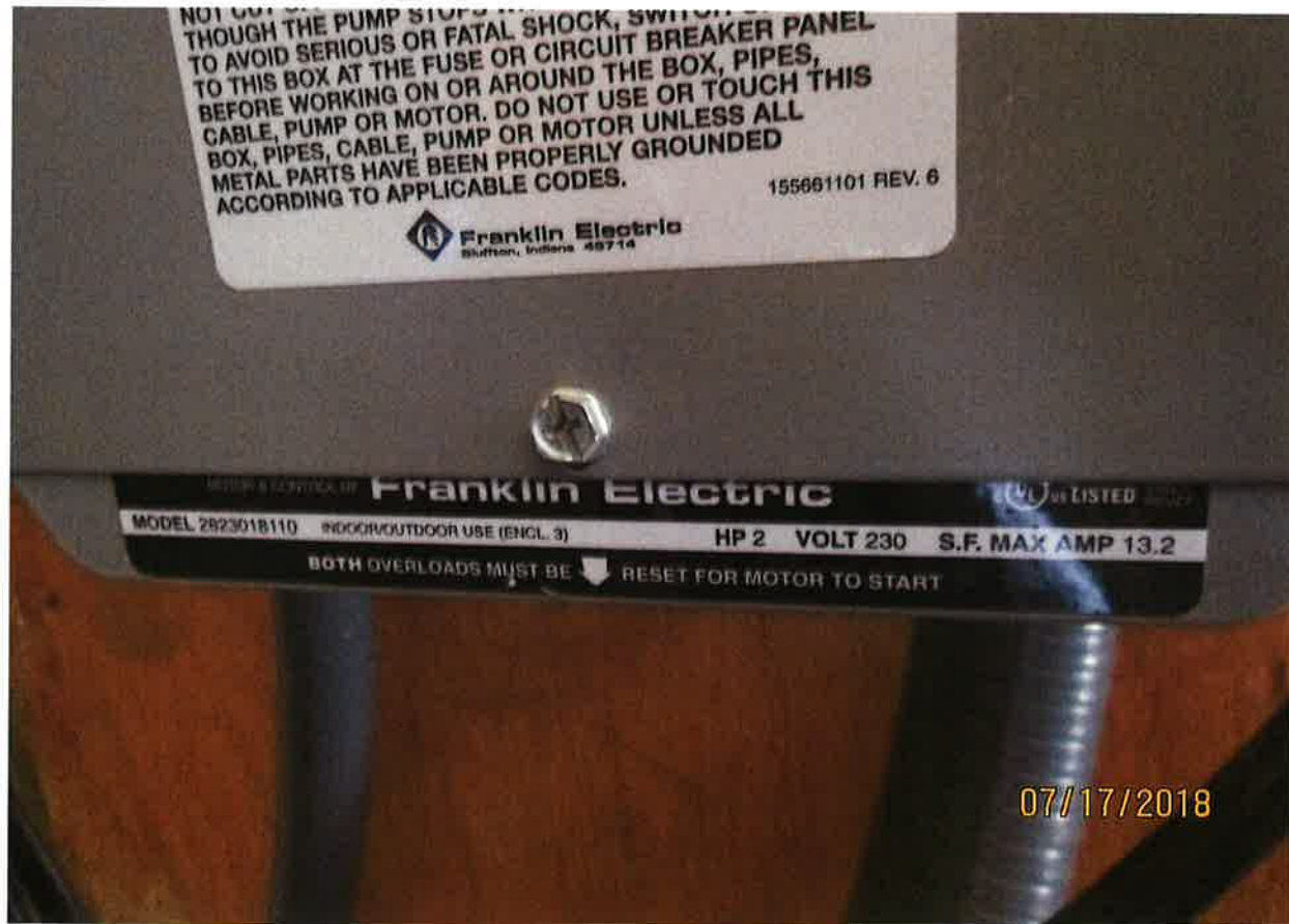
2hp Franklin pump in well.
