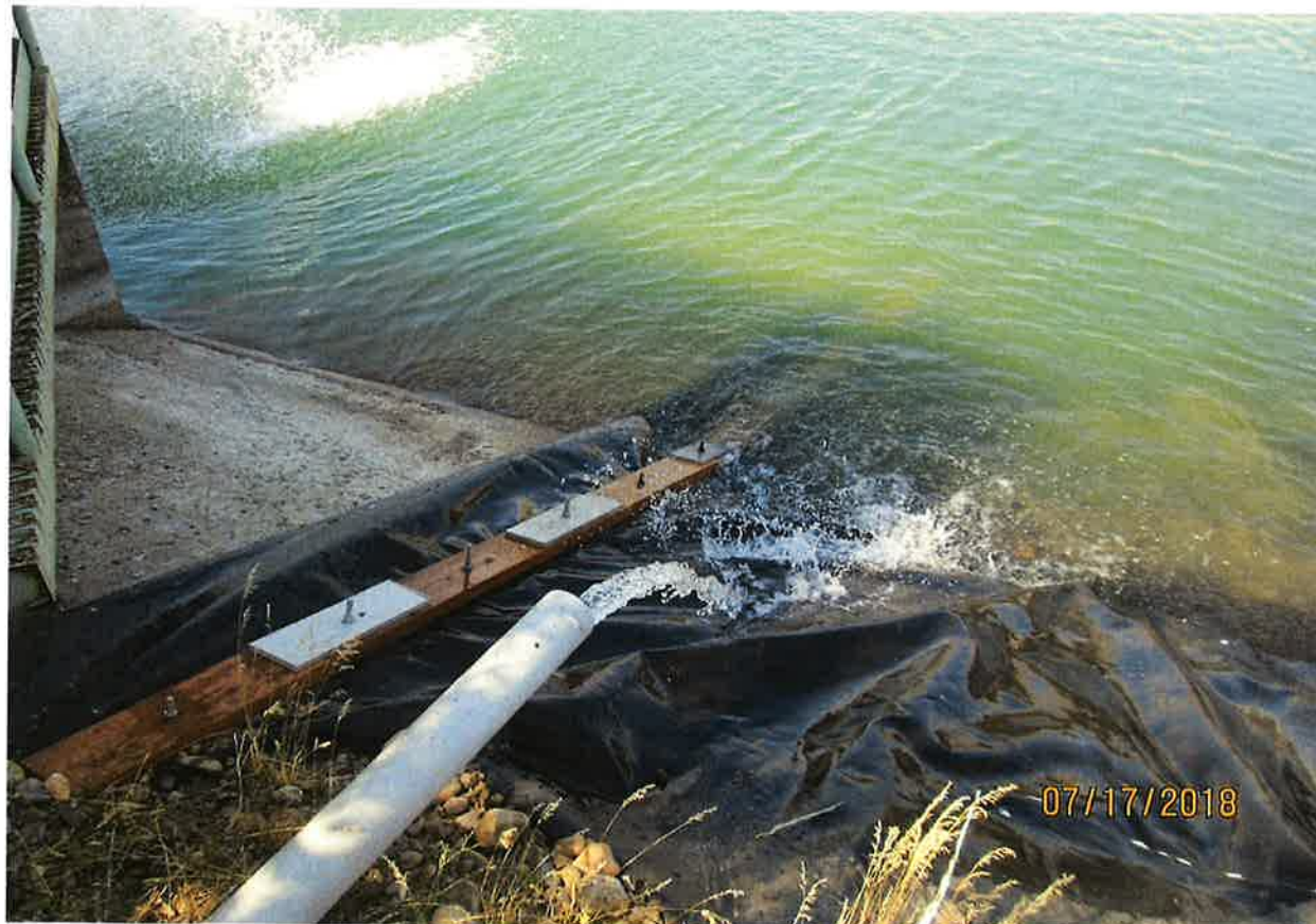
Water filling storage from well.
