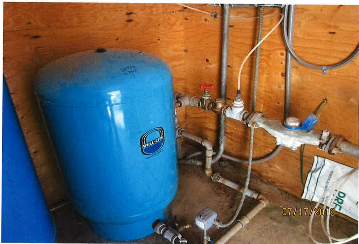
Inside of pump room. Unfortunately meter on system was from pressure tanks.
