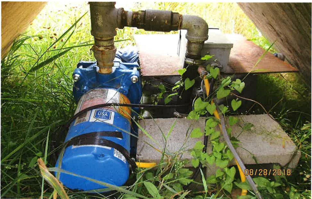
Applicant had installed a stilling well system to creek so sediment would not clog pump.
