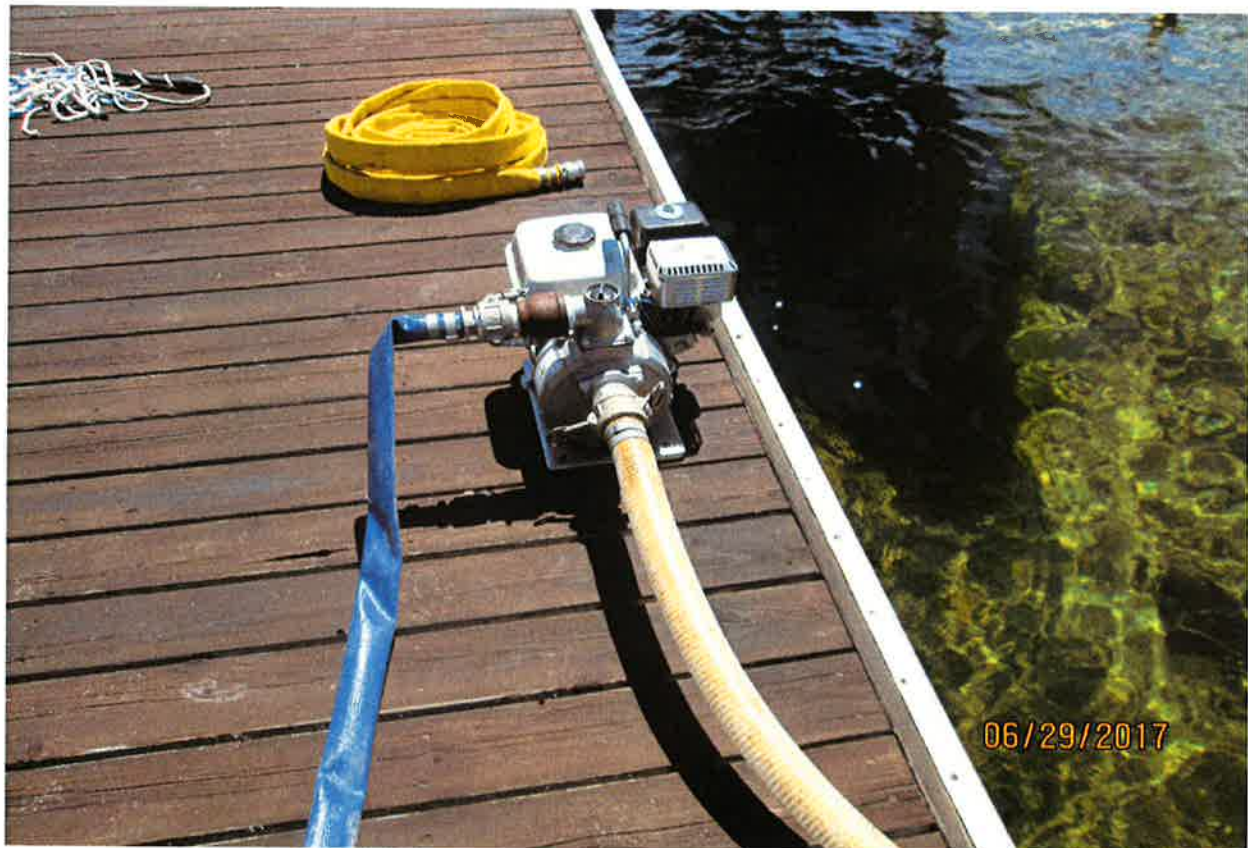
Applicant had separate pump for fire protection only. Amendment of Permit will add a 2 nd POD for fire pump.
