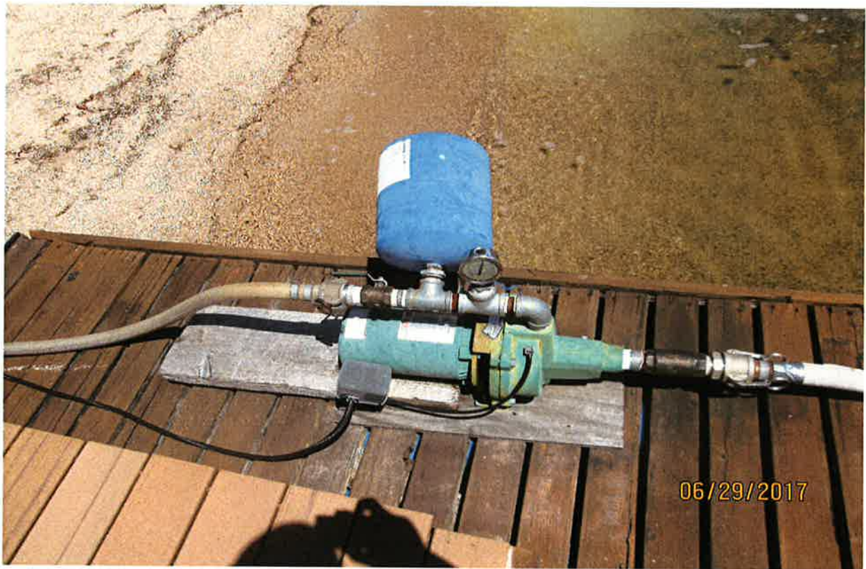
Pump on dock.
