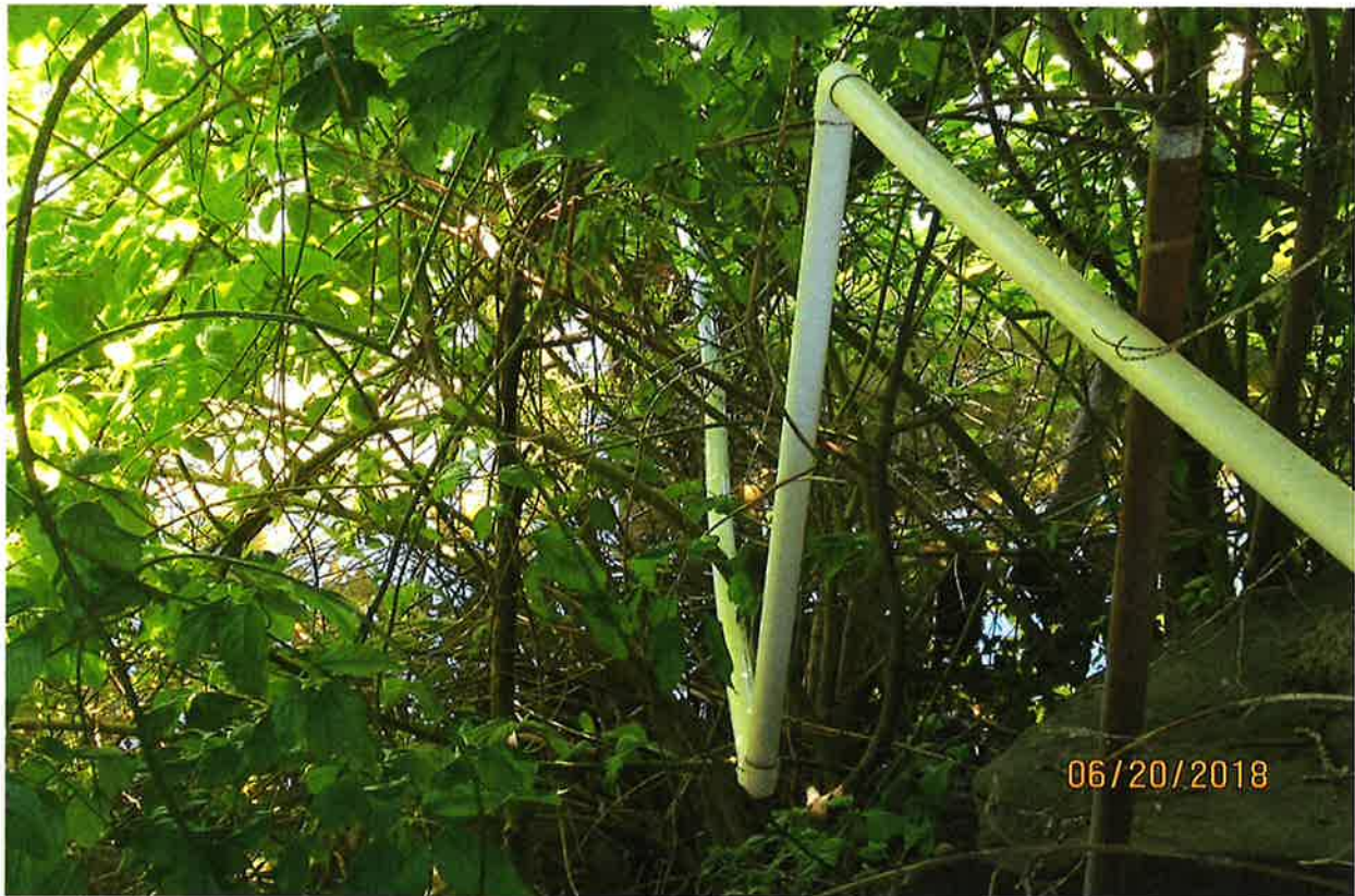
Pipeline from river to pump.
