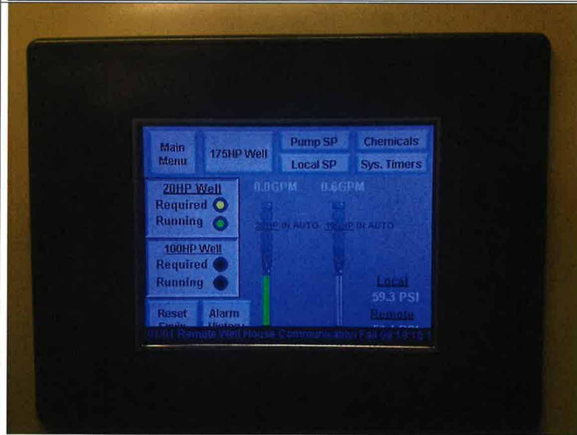
Automation system used to adjust flow, water quality chemicals, and visualize pump use.
