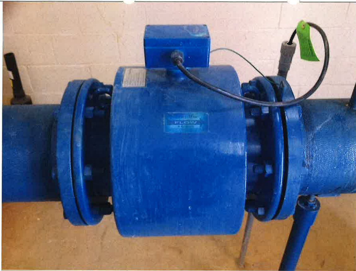
Ultra Mag flow meter connected to this well.
