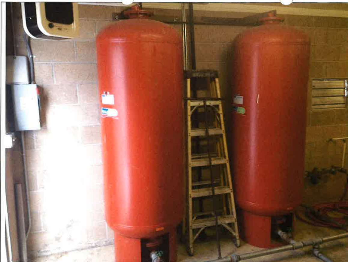
Pressure tanks used to alleviate spikes in the domestic system.
