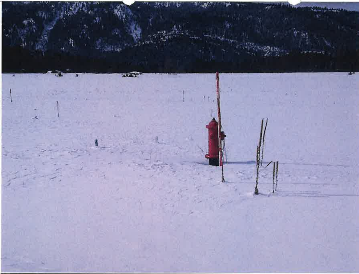
2 of 14 fire hydrants located in the Fire Protection POU. This one borders the undeveloped commercial use on the west side of Timberline Road.
