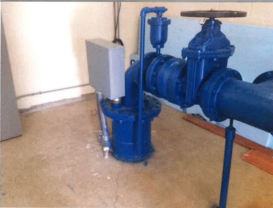
One pump is located in this well; a Karlington Electric 175 hp motor used for fire protection.
