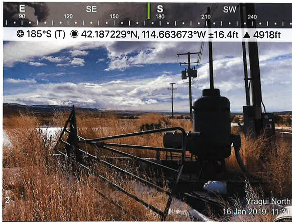
Figure 1: Point of diversion and pipeline to irrigation pond
