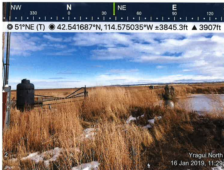
Figure 2: POD; lift pumps and irrigation pond
