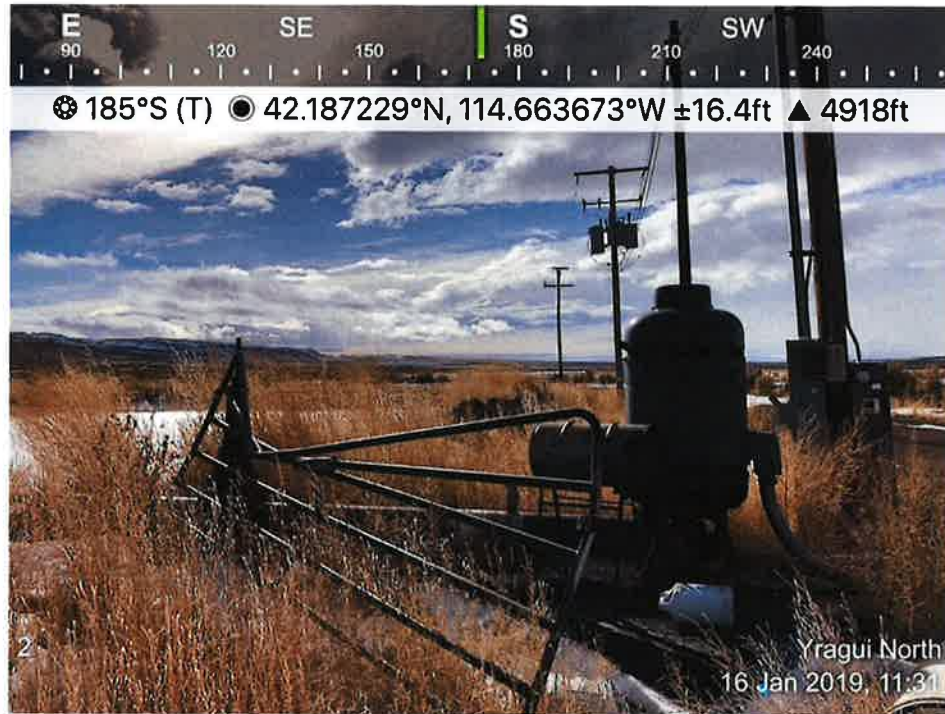
Figure 1: Point of diversion and pipeline to irrigation pond
