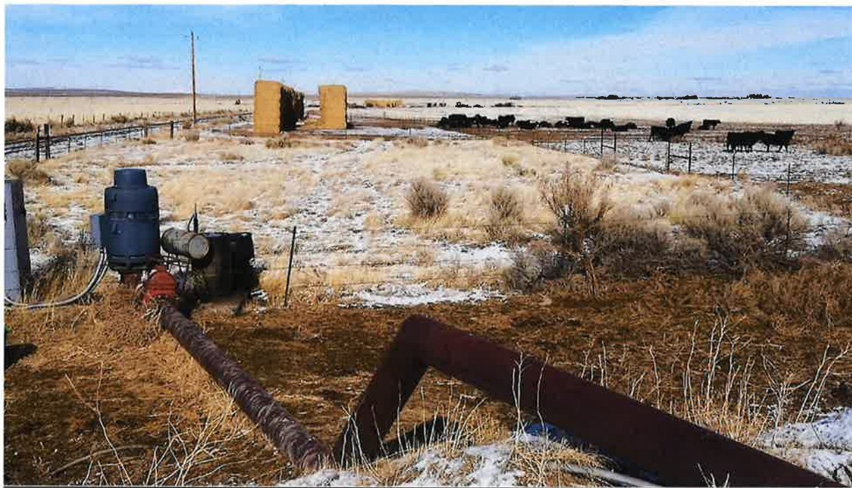
Figure 2: POD and pipeline to irrigation/stockwater pond
