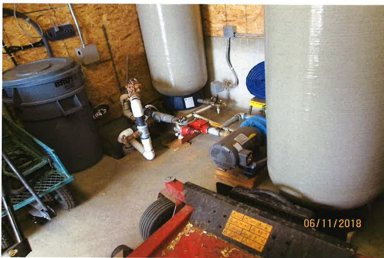
Pressure tanks and booster pump from reservoir.
