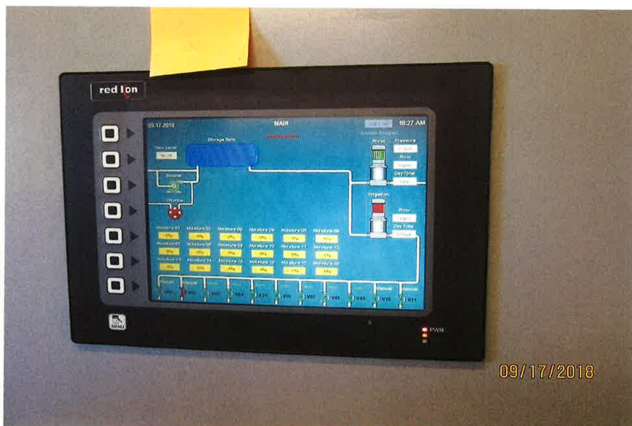
Irrigation system control panel.
