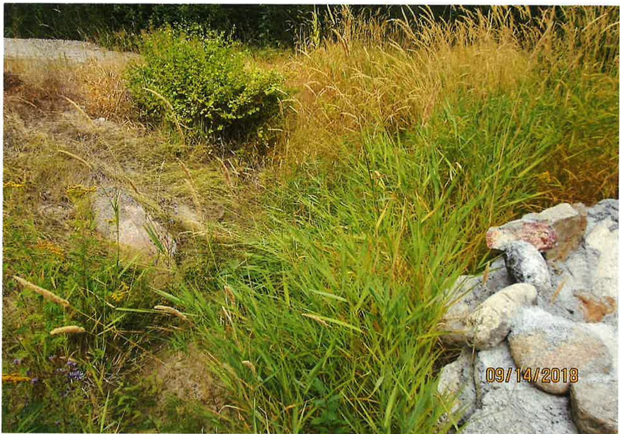
Build-up of sand and sediments and grasses in settling pool.
