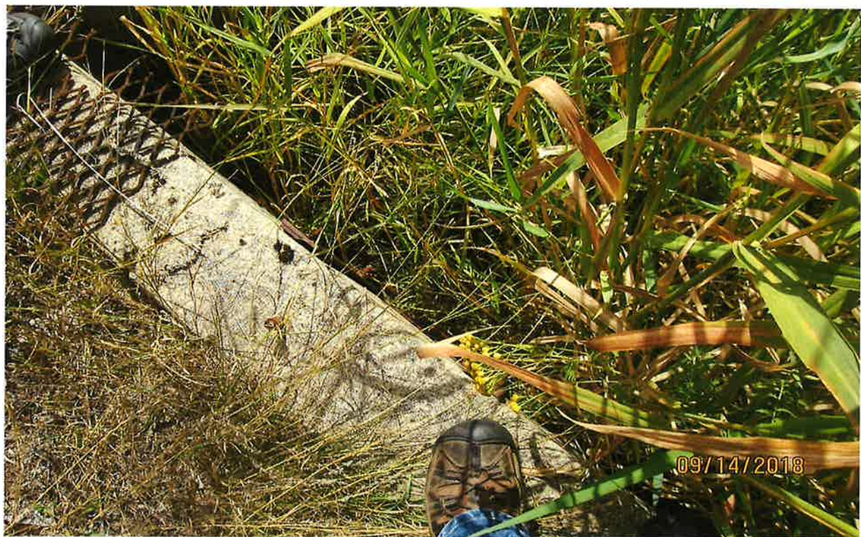
6 inch intake from settling pool to pond.
