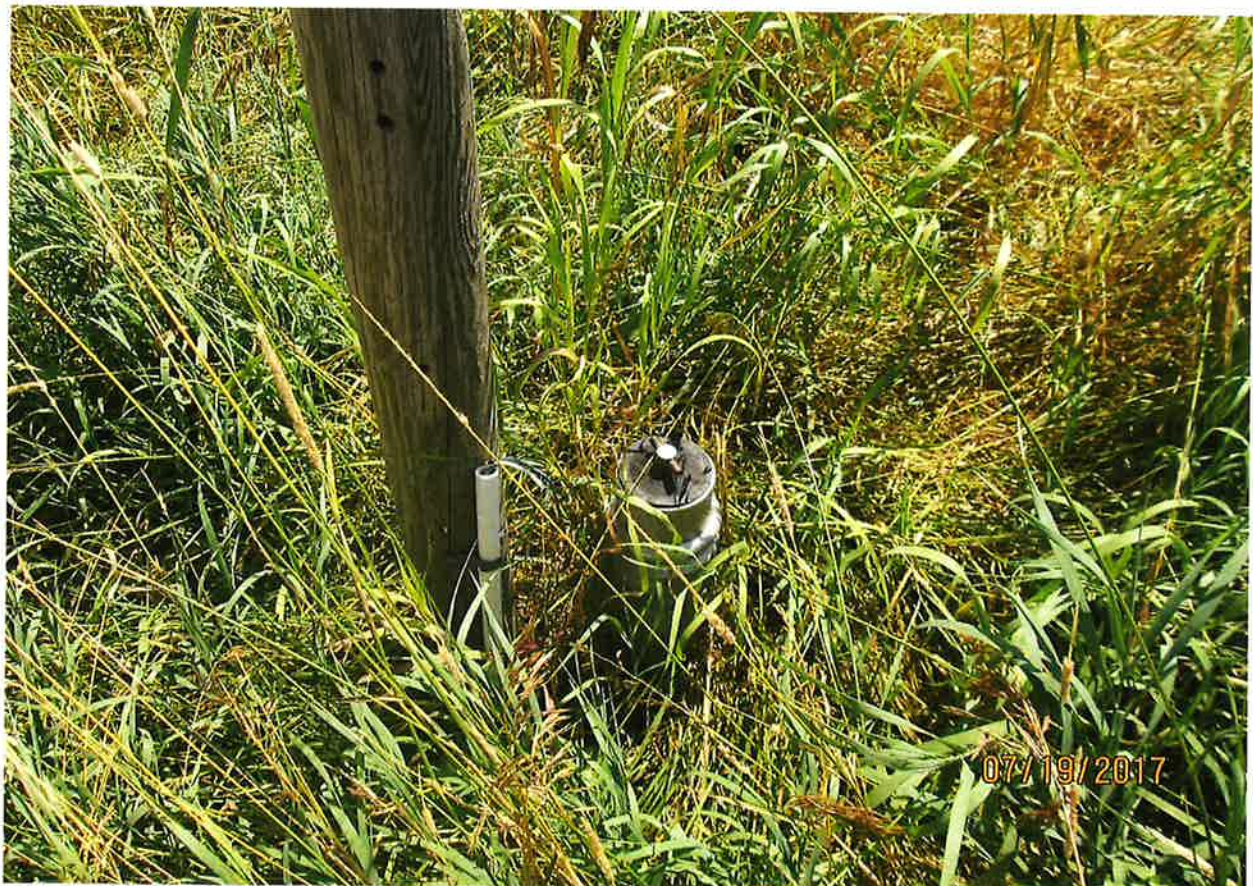
Another riser along main line.
