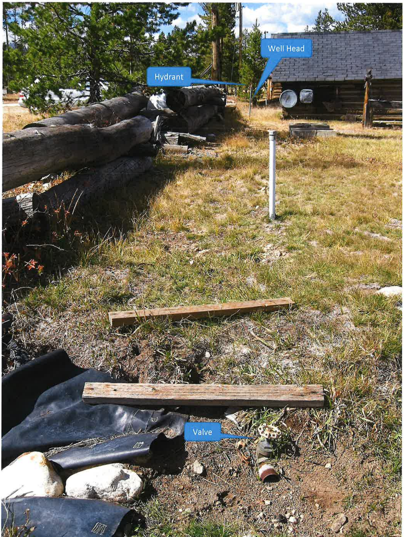
View from Valve to Well Head
