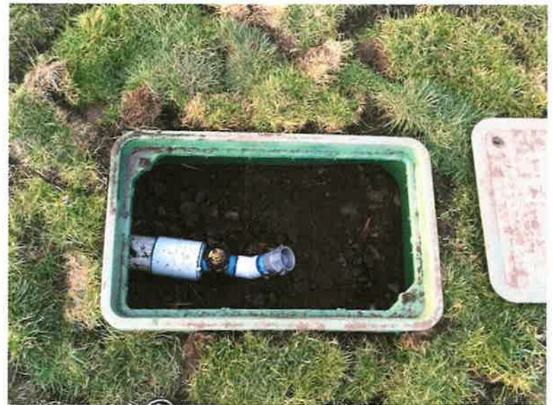
2-INCH CONNECTION FOR IRRIGATION
