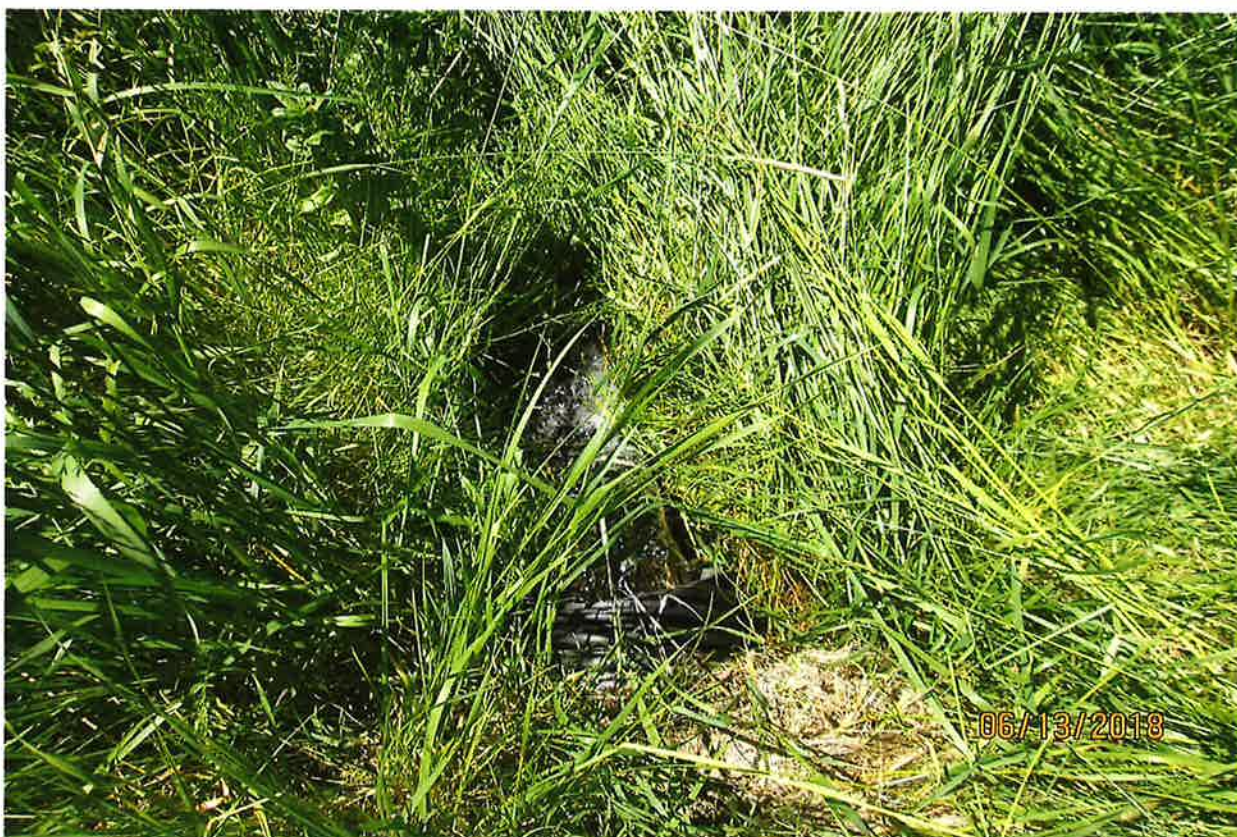
Return flow to creek. 6 inch pvc pipe.
