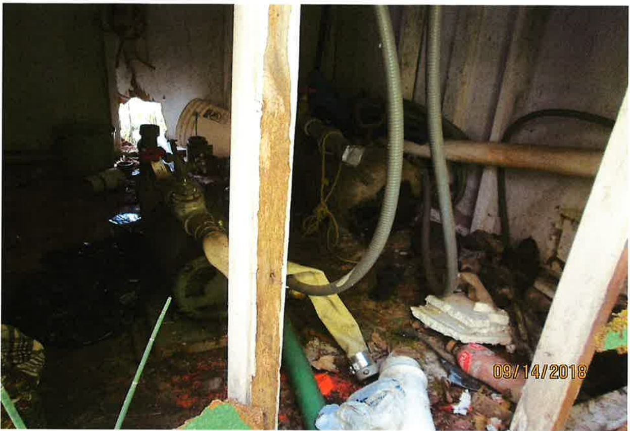
View of pumps through giant hole in pump house. Pumps looked in bad shape and didn't even work.
