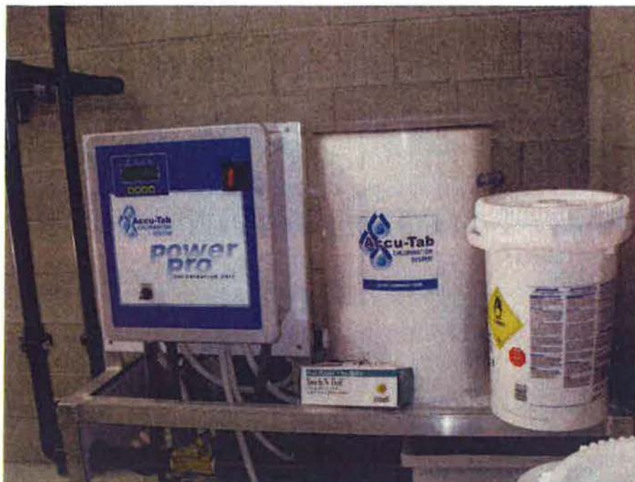
Figure 17. Tablet Chlorination System, Looking South
