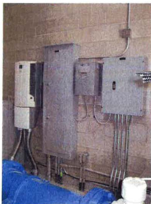
Figure 18. Controls, Looking Northwest
