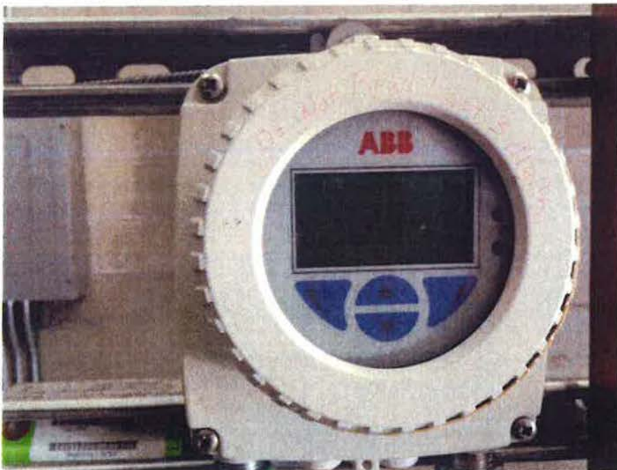
Figure 10. Flow Meter Reading #3, Approaching Peak Flow
