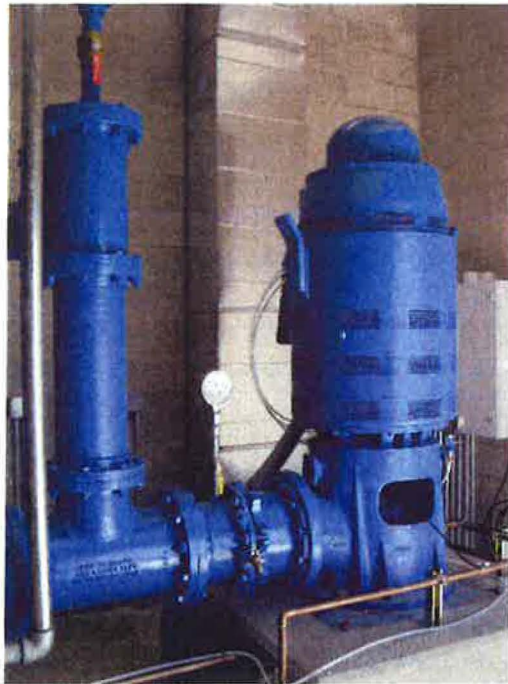
Figure 4. Well No. 20 Vertical Turbine Pump and Motor
