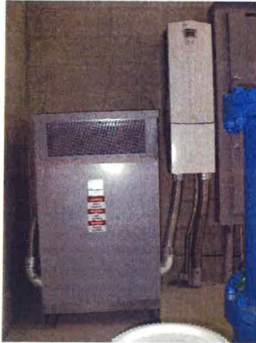
Figure 19. Controls, Looking North
