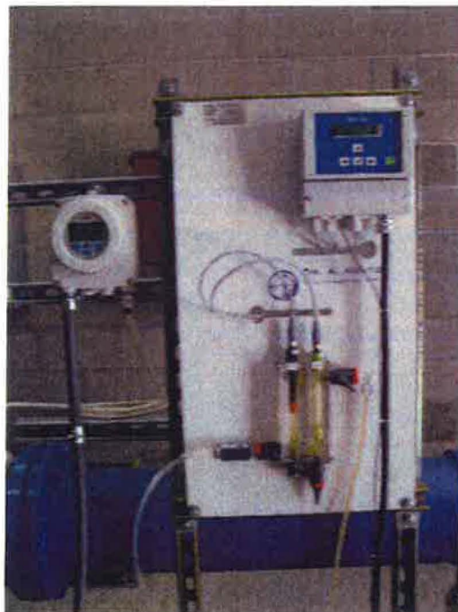
Figure 16. Flowmeter and Chlorine Analyzer, Looking North
