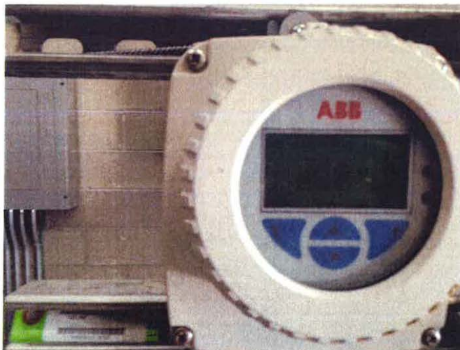
Figure 8. Flow Meter Reading #1, Approaching Peak Flow
