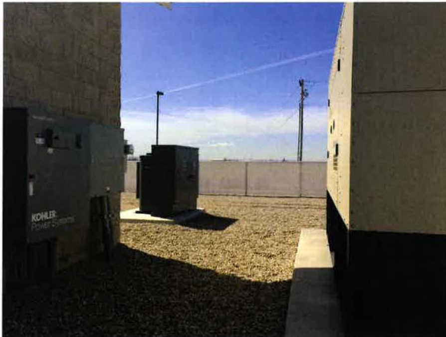
Figure 2: North Side of Well House with Transformer, Backup Generator, & ATS, Looking West
