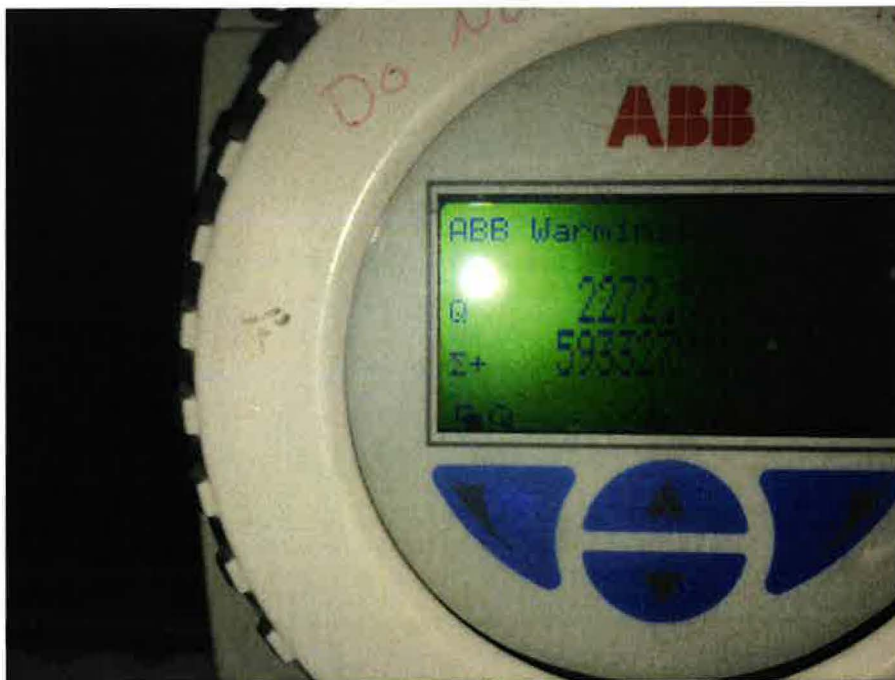
Figure 14. Flow Meter Reading #7, Approaching Peak Flow
