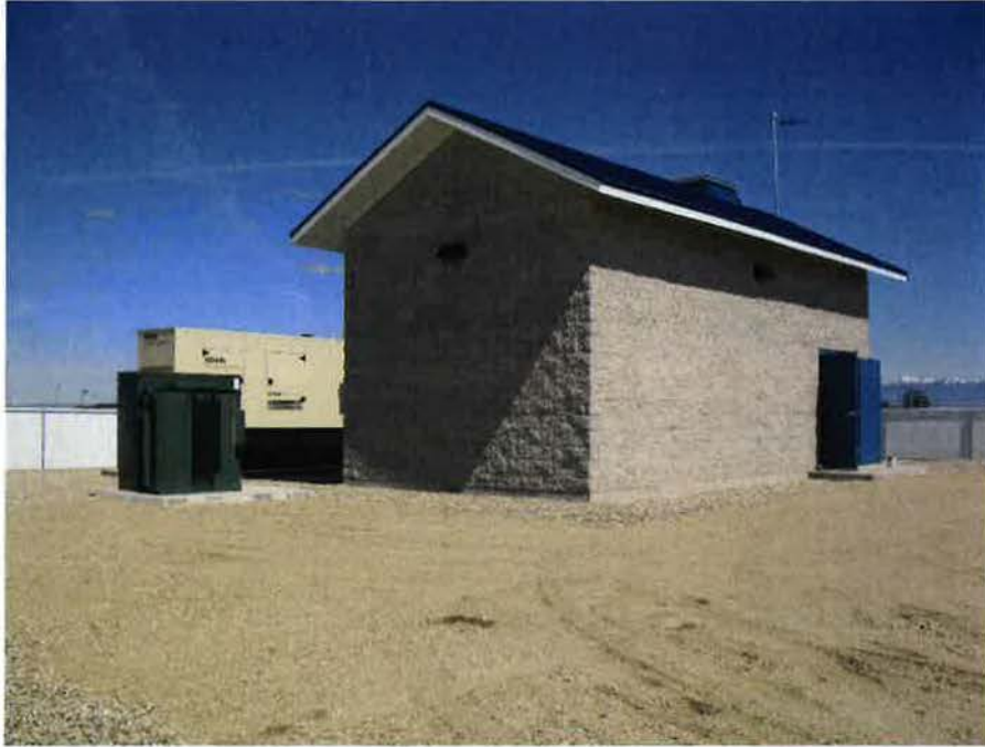
Figure 1. Housing for Well No. 20 with Transformer and Backup Generator, looking Northeast
