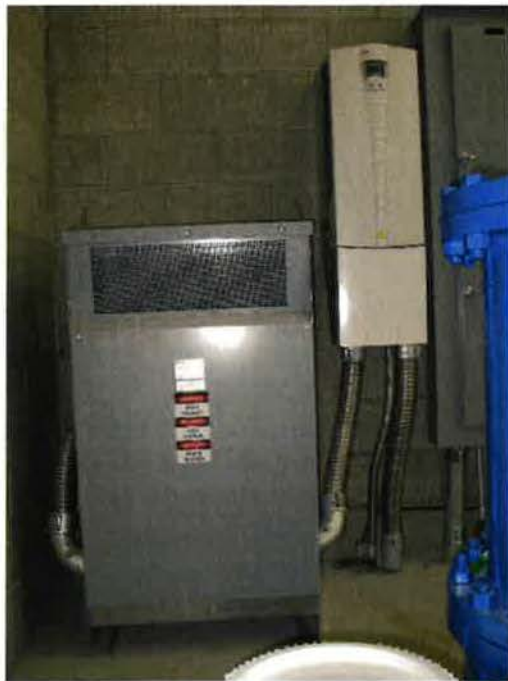
Figure 19. Controls, Looking North
