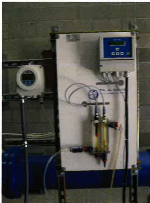
Figure 16. Flowmeter and Chlorine Analyzer, Looking North
