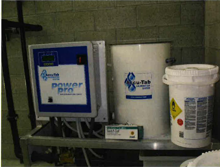
Figure 17. Tablet Chlorination System, Looking South
