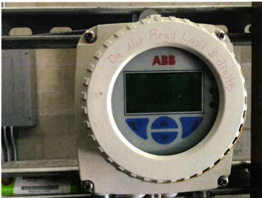
Figure 10. Flow Meter Reading #3, Approaching Peak Flow
