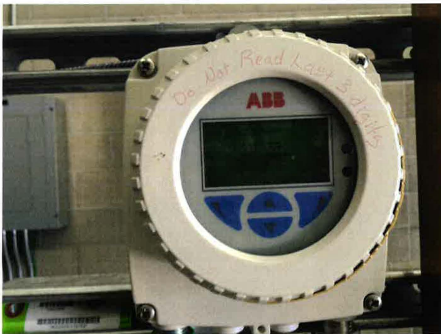
Figure 12. Flow Meter Reading #5, Approaching Peak Flow
