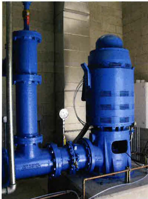
Figure 4. Well No. 20 Vertical Turbine Pump and Motor
