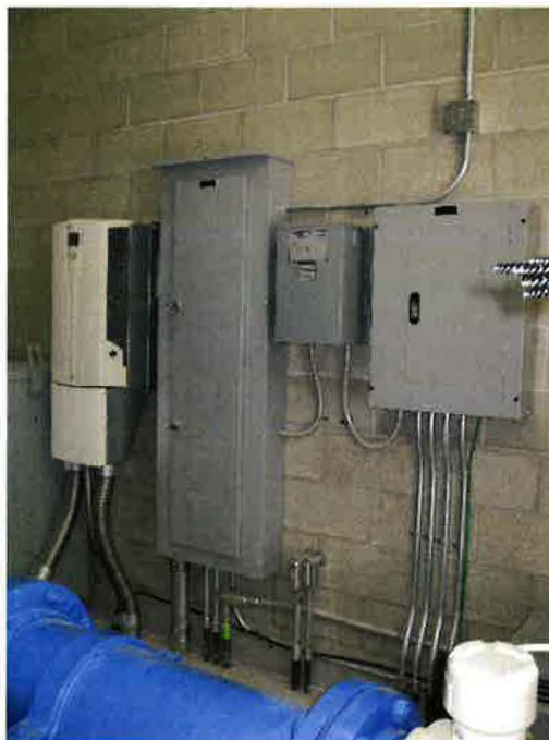
Figure 18. Controls, Looking Northwest
