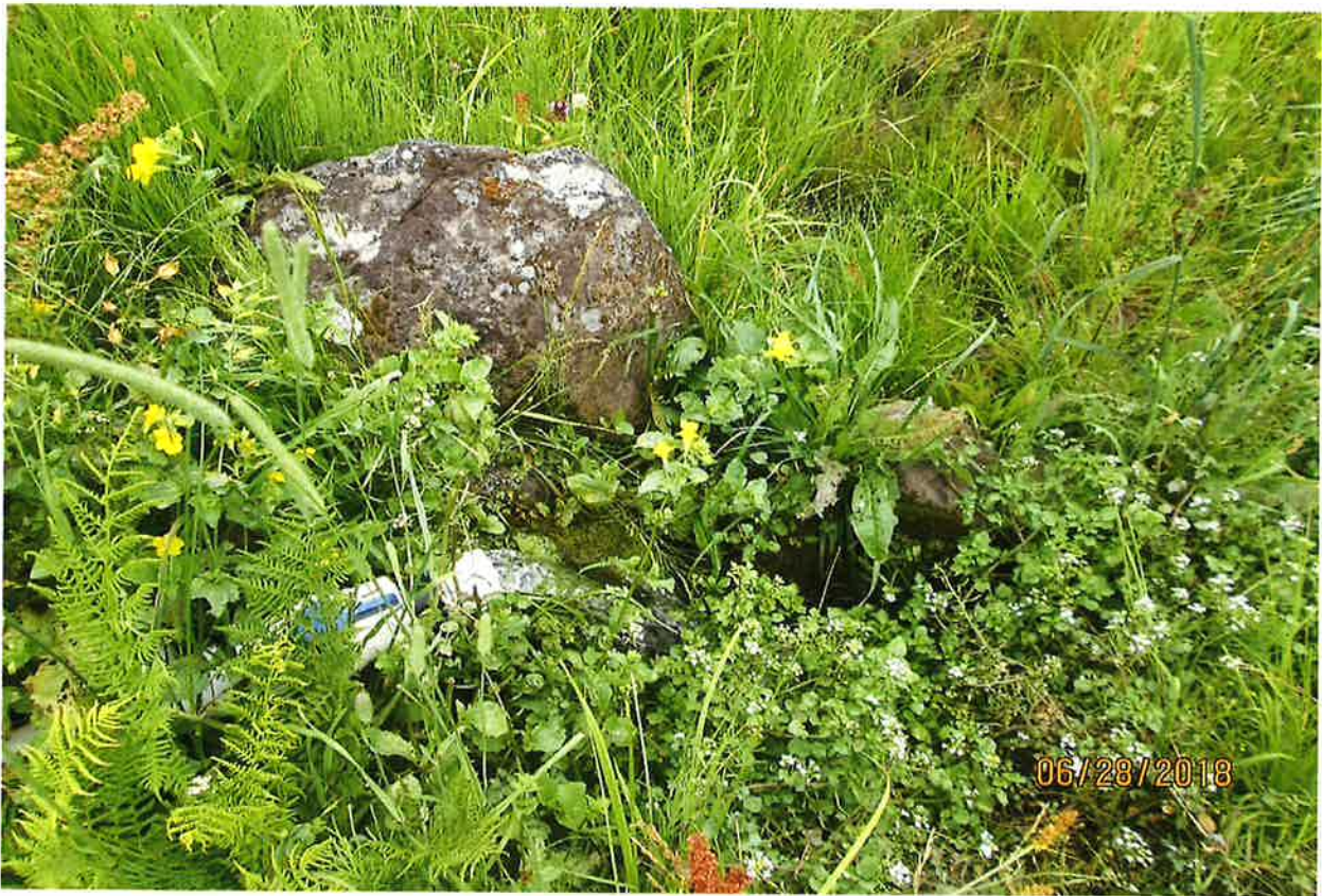
Diversion pipe from groundwater source used for stockwater and irrigation. 5 gallon bucket test performed and filled in average of 7.8 seconds which is equal to 38.5 gpm or 0.09 cfs.
