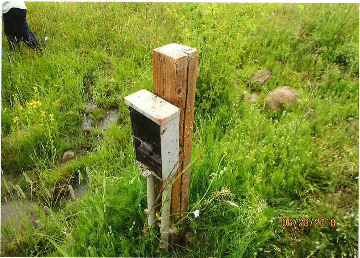
Unknown pump size electrical box next to culvert.
