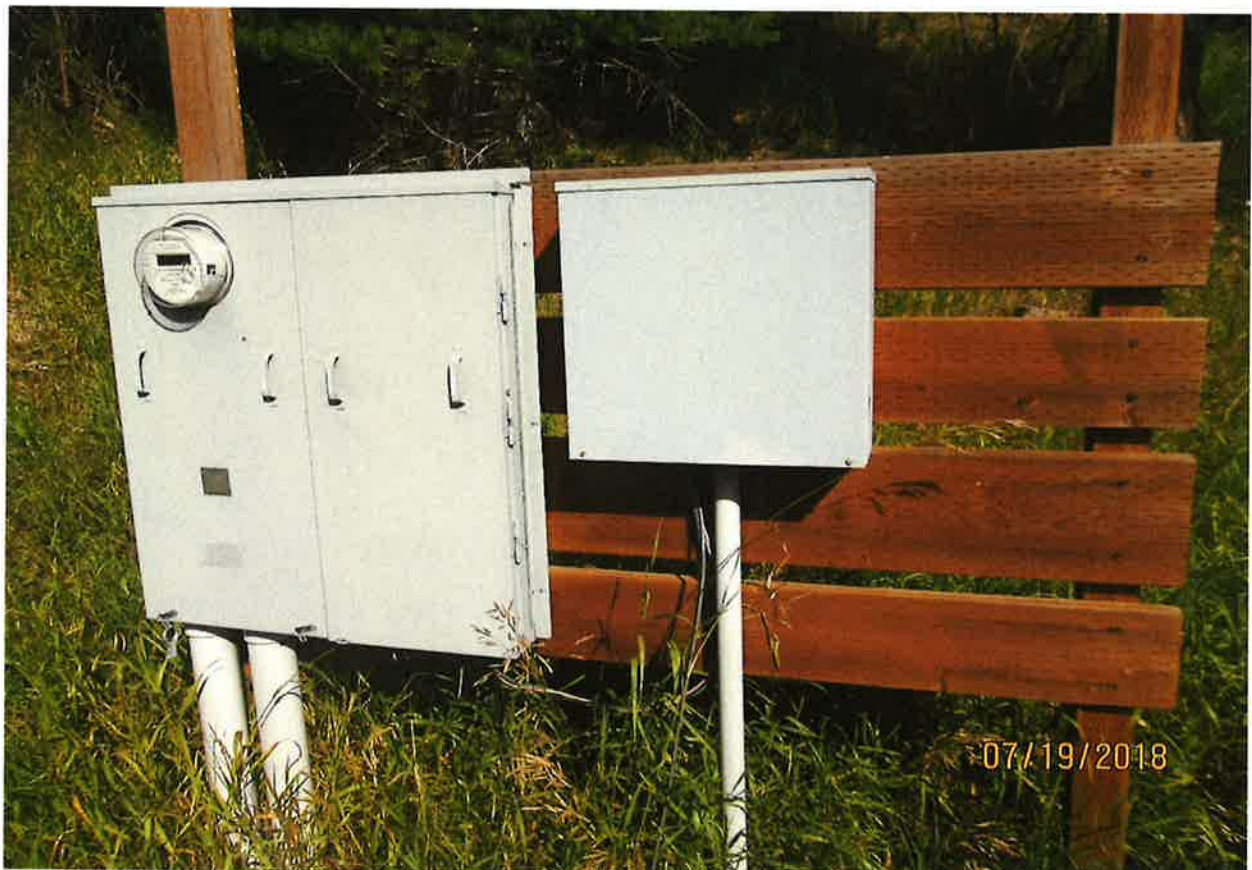
Power and pump box. Well was equipped with unknown pump size.
