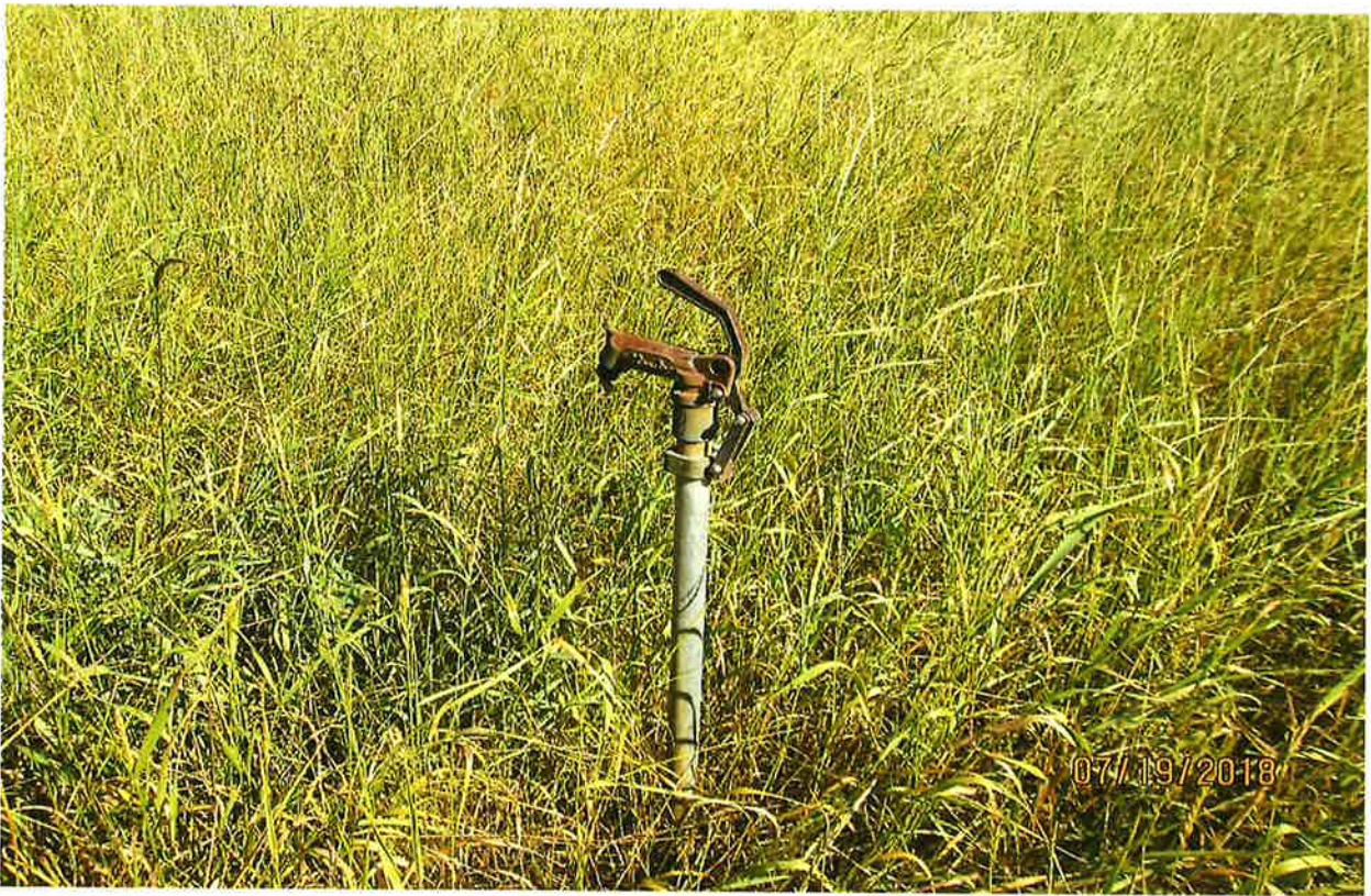
Frost free hydrants placed around property.
