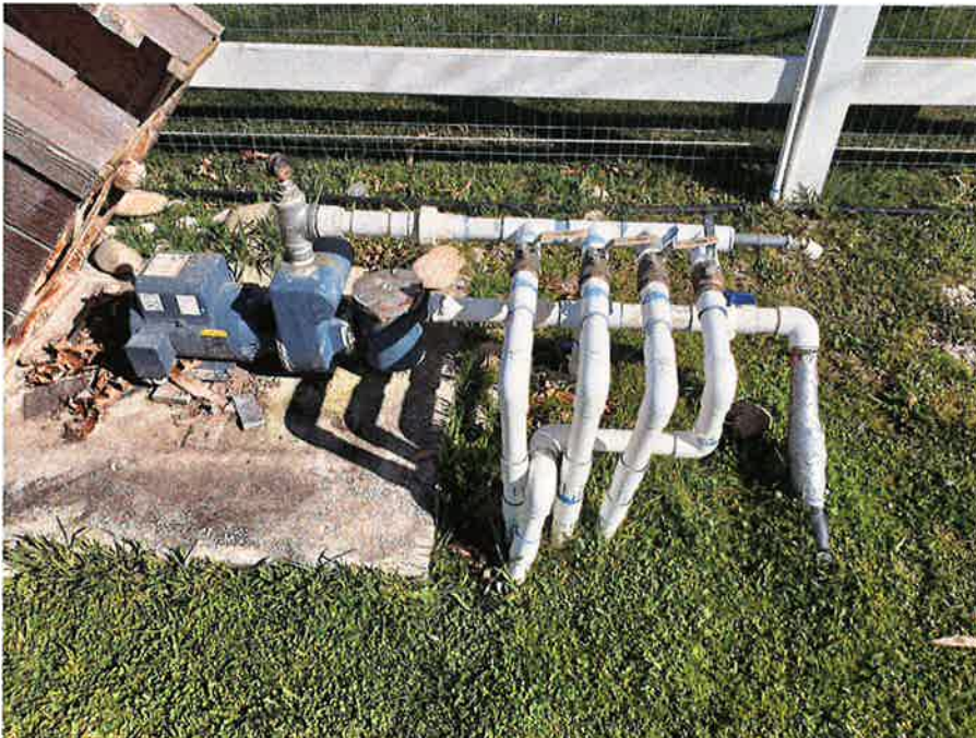
Figure 2 A 5-hp pump used to divert water from the pond to the irrigation system.
