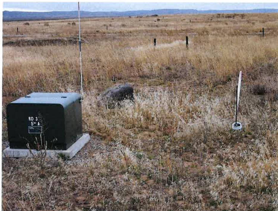
Figure 4: A stub-out with a marker and with additional markers in the background
