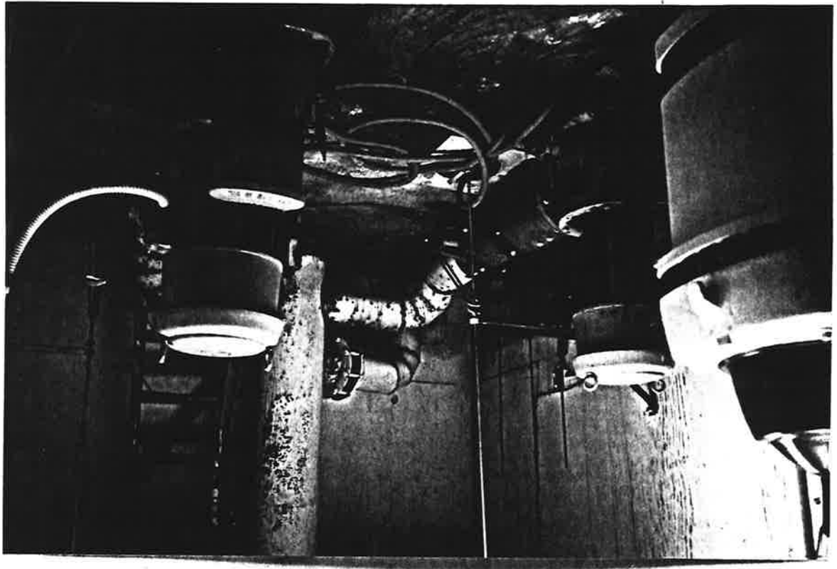
Inside of Shed with distribution pumps
