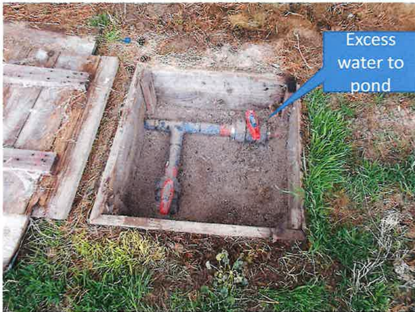
Valve Box that controls water to house
