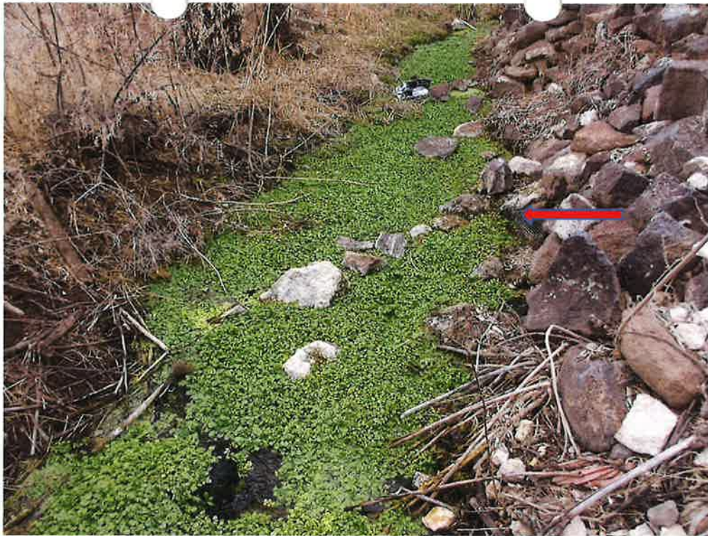
POD (at arrow) on unnamed stream. Pipe is partially submerged and obscured by a trash screen and aquatic vegetation. Note rock wing dam across stream.
